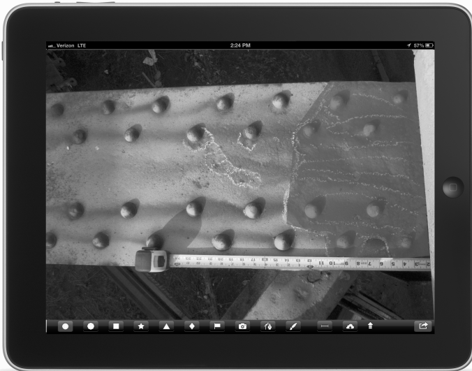
Figure 2. Digital photo taken in the field with a freehand drawn annotation, which shows deteriorated area of a cover plate.
