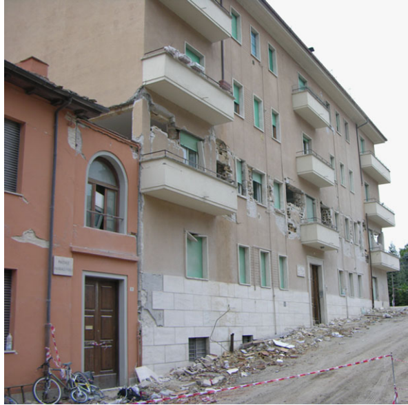
Fig. 1 Damage of a four-story conventional building due to pounding with its adjacent two-story building, during the L'Aquila earthquake in Italy, in April 2009 [8]
