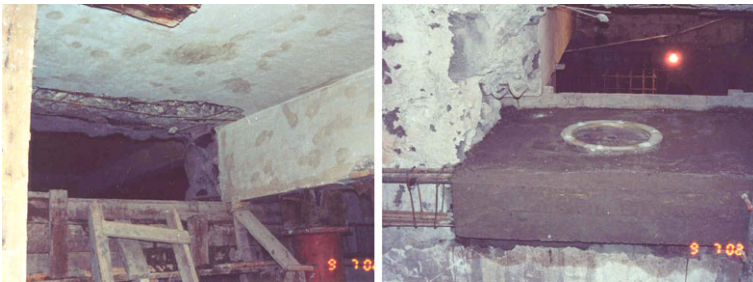
Fig. 12 Existing beam is crossing the space of the opening and supported by temporary columns
