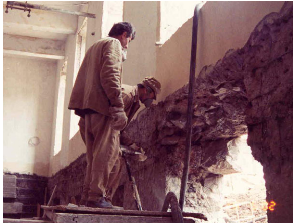
Fig. 8 Retrofitting of existing 3-story stone school building: the case when the opening has the part of the existing wall above it
