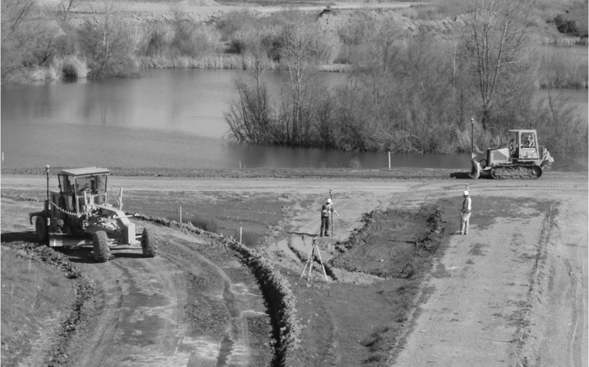
Figure 15.6 A dozer and grader using machine control to create an intersection of roads. (Courtesy Topcon Positioning Systems, Inc.)
