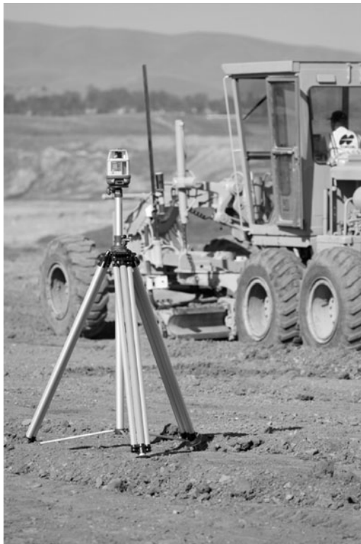
Figure 23.2 Rotating laser providing finished grades to machine control system in grader. (Courtesy Topcon Positioning Systems.)
