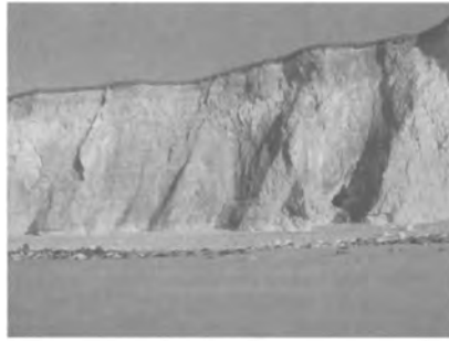
Quiberville, Newhaven Chalk, steeply inclined conjugate joints (pyramidal structure)
