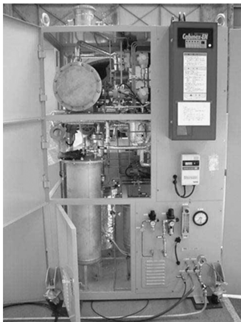
Figure 15.16 IPA purification plant using vapor permeation with A-type zeolite membranes
