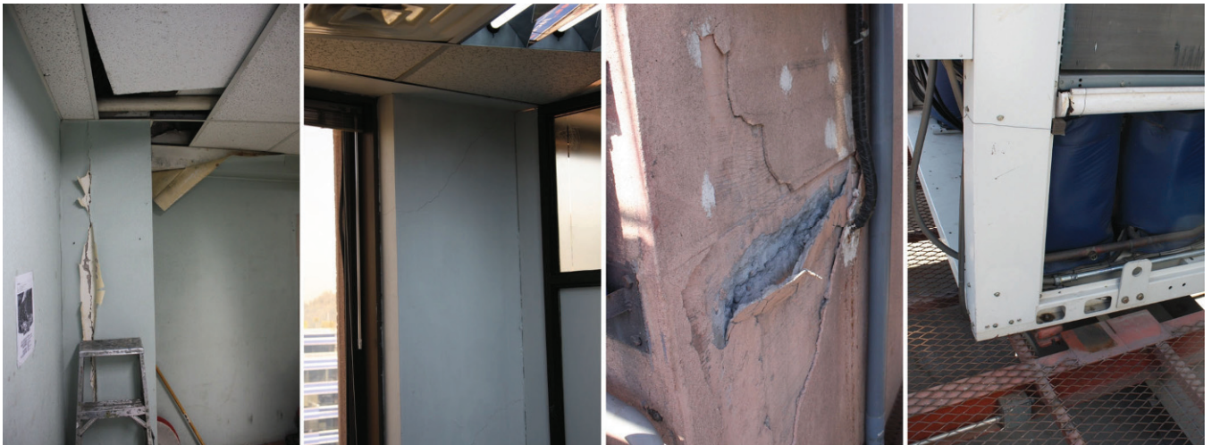
Fig.8 Observed damage after the 2010 Chile Earthquake
