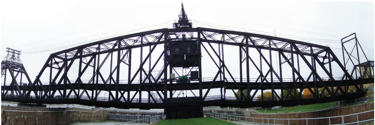
Fig. 2 Span II of the Government Bridge in its locked position to allow rail and vehicular traffic
