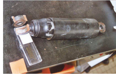
Fig. 2 Broken Dampers device of Iroise Bridge (FR)
