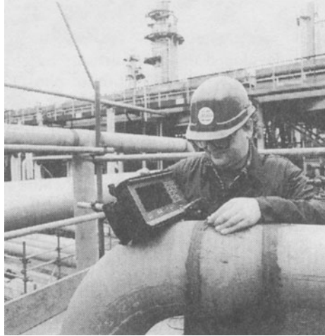
Figure 5.13 Ultrasonic inspection of butt welds in a pipe (Courtesy of Wells-Krautkramer Ltd)
