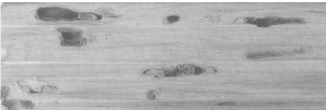
Figure 9.1 Worm damage in imported maple flooring
