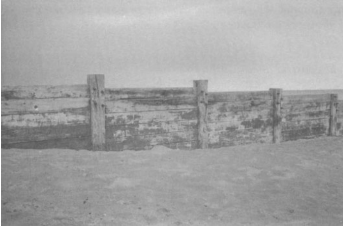
Figure 10.5 Timber groynes for control of littoral drift
