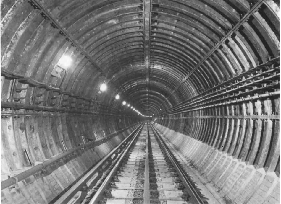
Figure 2.3 A running tunnel constructed with bolted cast-iron linings. Tunnel diameter is 3.8 m, suitable for small rolling stock
