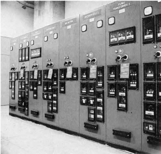
Figure 21.5 Medium-voltage switchgear room
