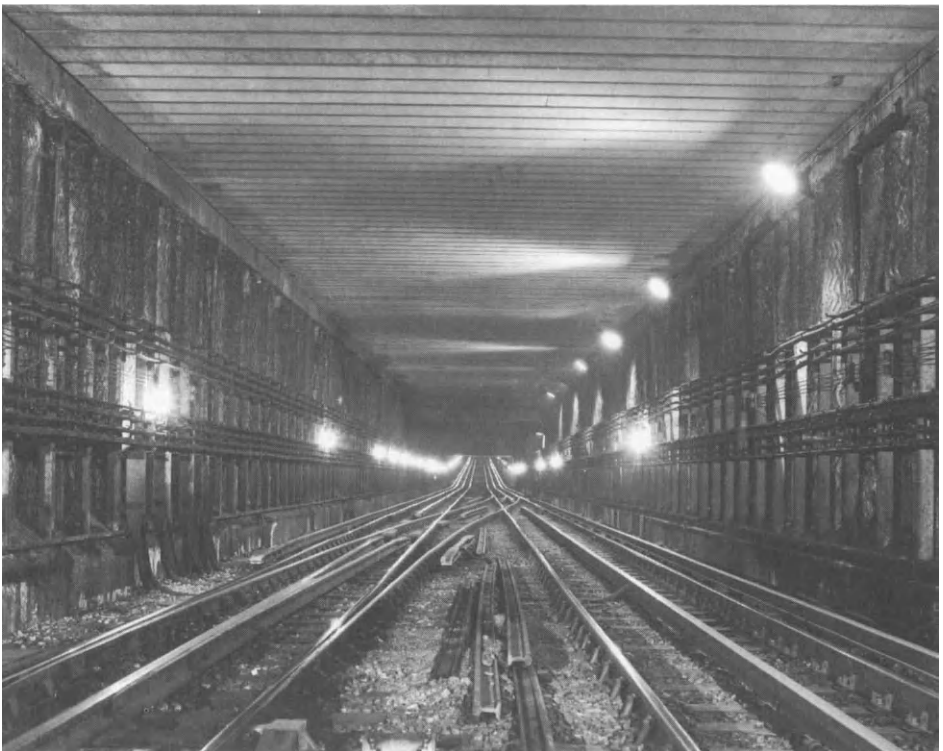
Figure 2.1 A typical covered way in concrete construction. The side walls are formed with continuous piles and the roof with precast beams. Dimension between side walls is approximately 7.3 m
