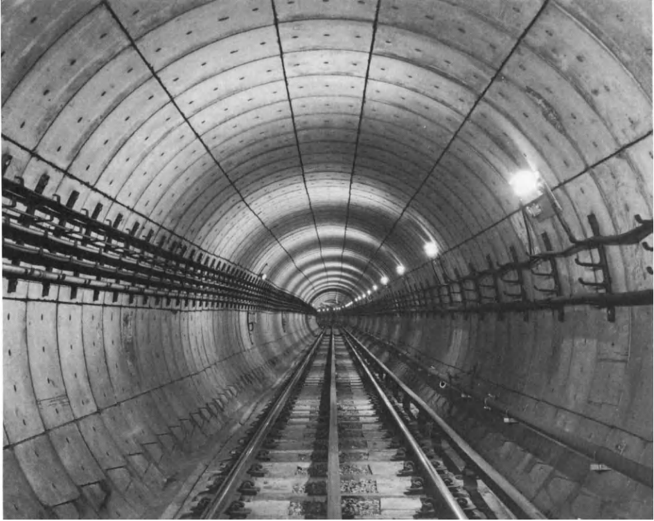
Figure 2.5 A running tunnel, 3.8 m diameter, constructed with expanded concrete linings. The wedges for expanding the rings can be seen on each side
