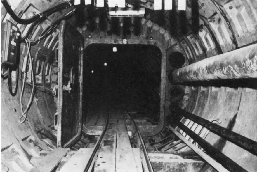
Figure 18.3 Airlock: water-transmission tunnel system, first-stage tunnels, for Metropolitan Works Authority, Bangkok, Thailand
