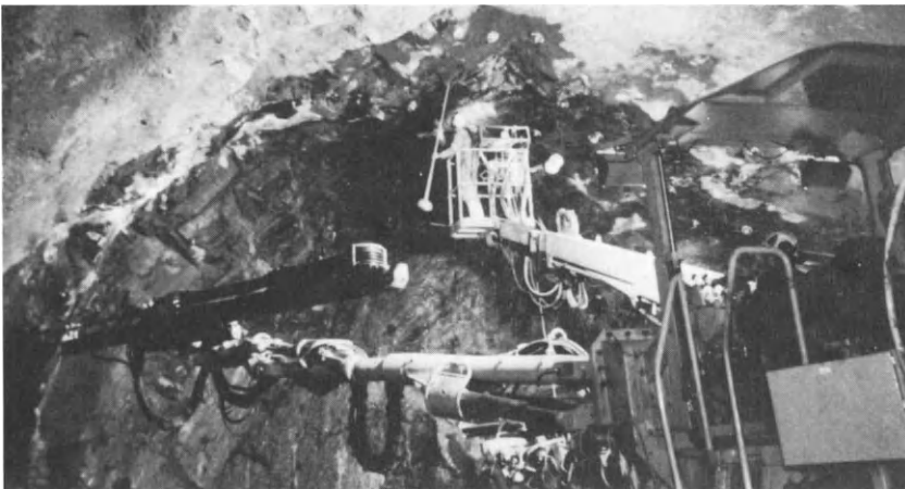
Figure 17.1 A modern drilling rig operating in a 68 m 2 tunnel (a rock bolt is being installed)
