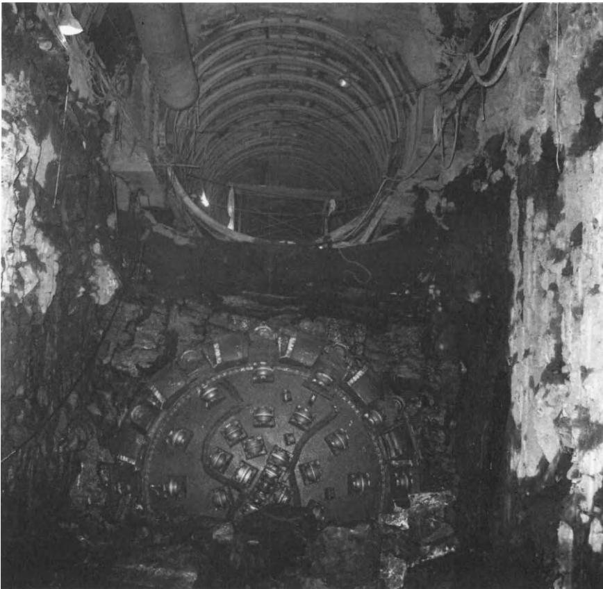
Figure 16.3 New York City 63rd Street Subway. Superimposed tunnels supported by steel ribs
