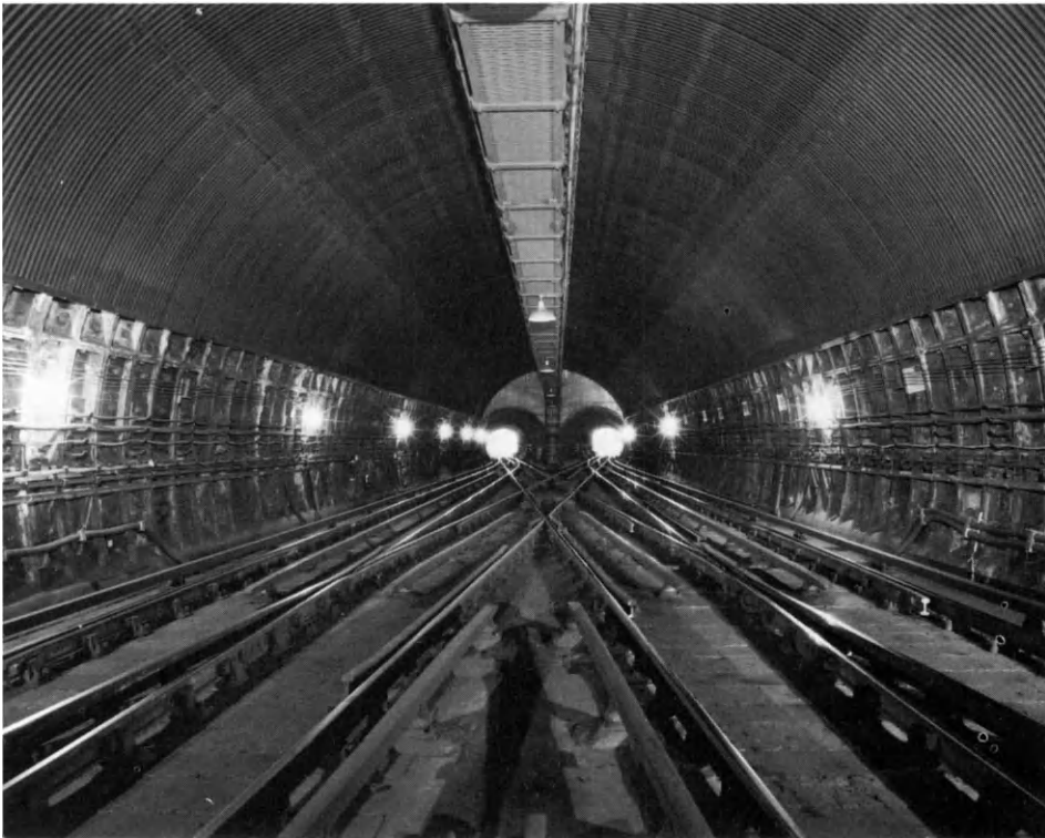
Figure 2.6 A 9.5 m diameter cast-iron lined tunnel providing space for a scissors crossover at a terminal station. The longitudinal high-level gantry carries the cables through the single tunnel. The secondary lining in the soffit directs seepage water to the sides where it is led away to the drainage system
