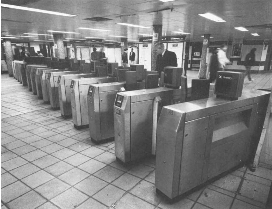
Figure 3.11 Ticket-operated entry and exit gates newly installed in the concourse of an existing station
