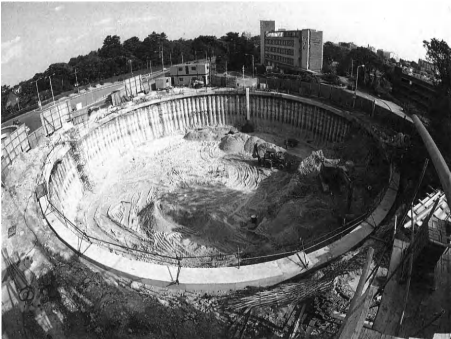
Figure 8.6 Use of capping beam and slender CFA piles to construct a circular access area in sands (courtesy Cementation Piling & Foundations Ltd)
