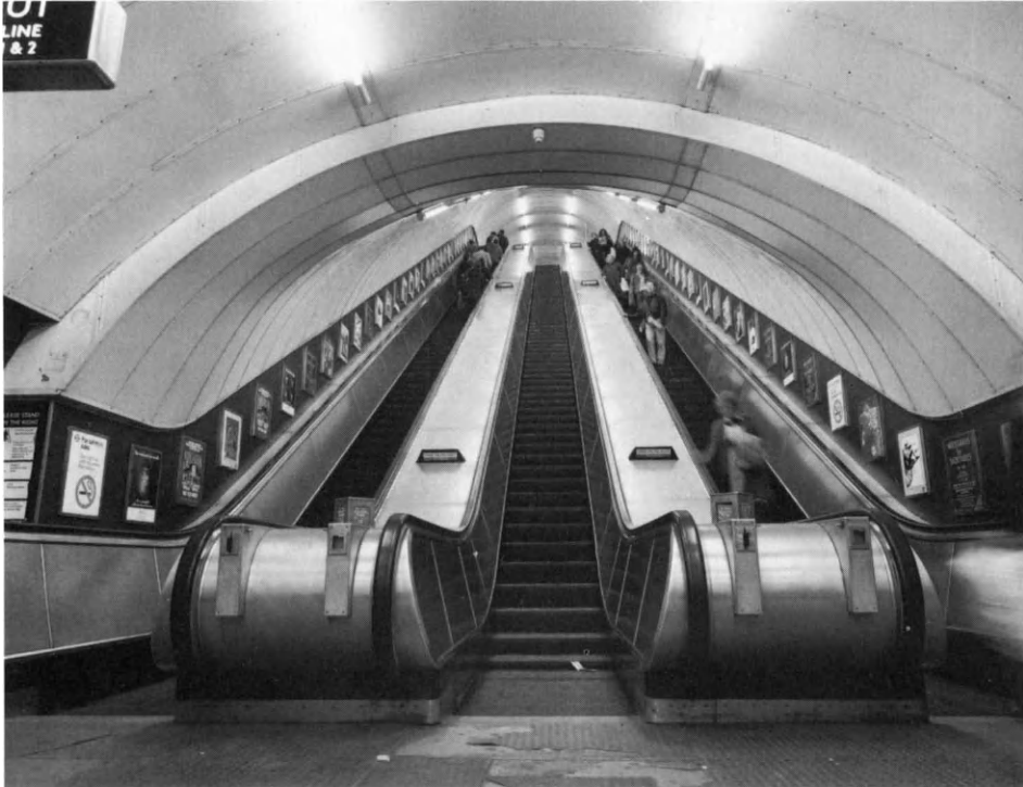
Figure 3.9 A set of three escalators accommodated within a 7.5 m diameter inclined shaft
