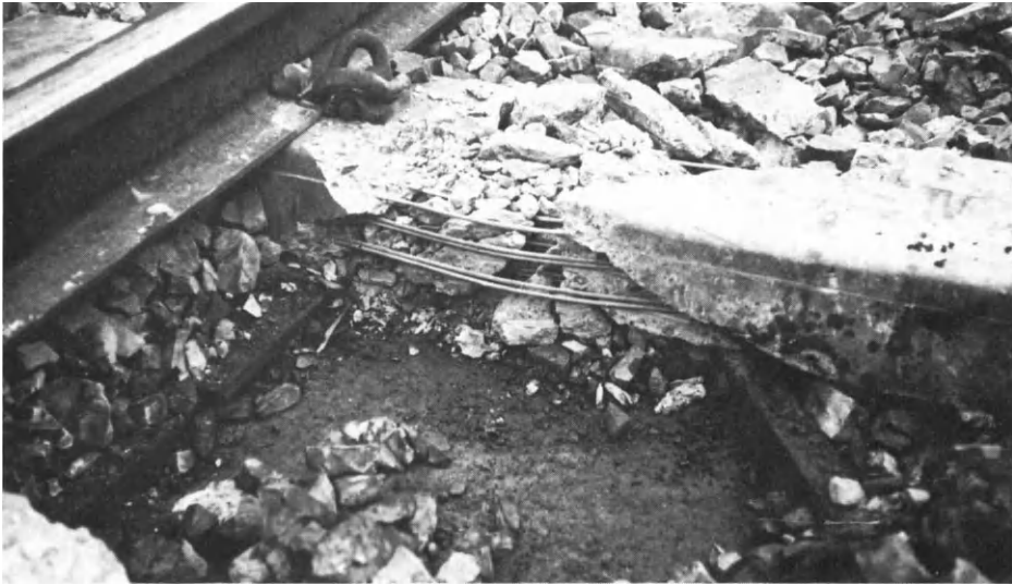
Figure 5.7 Derailment damage to a concrete sleeper
