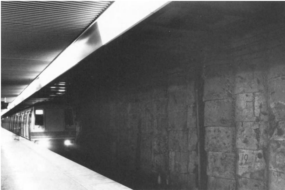
Figure 9.8 Caisson wall exposed in completed station structure. The HDC linings have been removed
