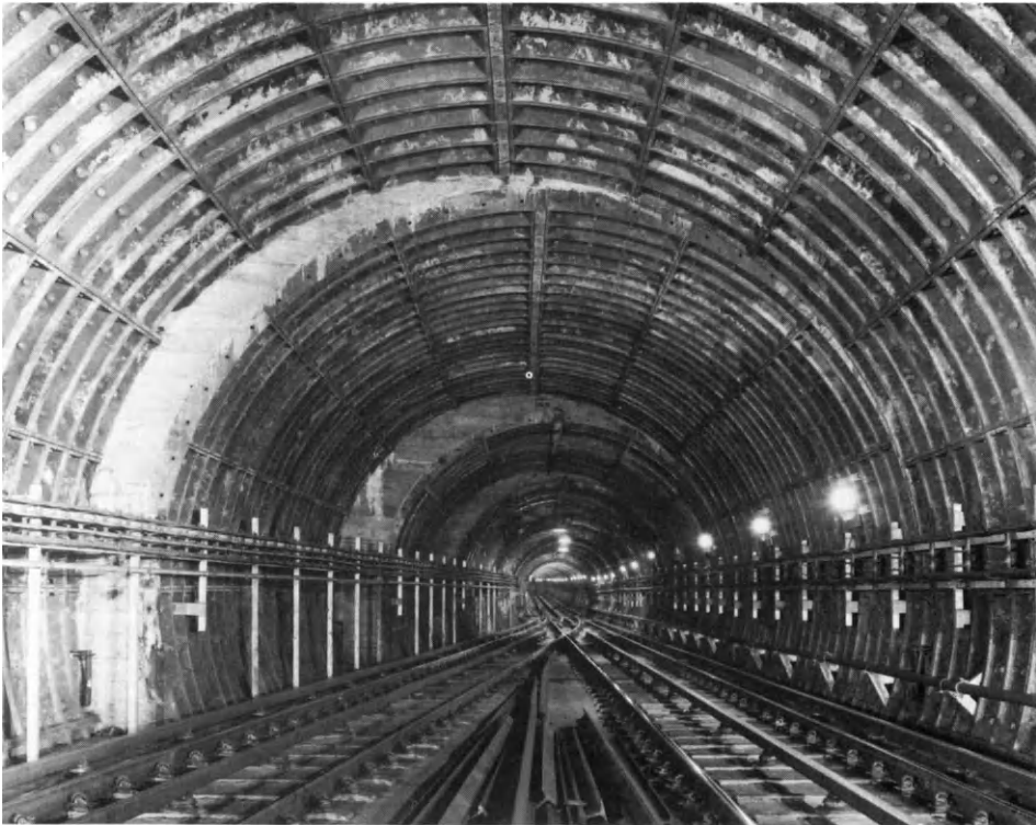
Figure 2.4 A step plate junction accommodating a simple turnout formed with bolted cast iron linings. The largest diameter (in the foreground) is 9 m and the smallest 3.8 m
