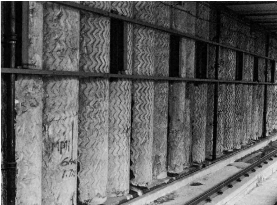
Figure 8.12 Use of true secant piling to form a reasonable quality finish requiring no facing – Hong Kong Metro (courtesy Lillbore – F. C. Lilley, UK)
