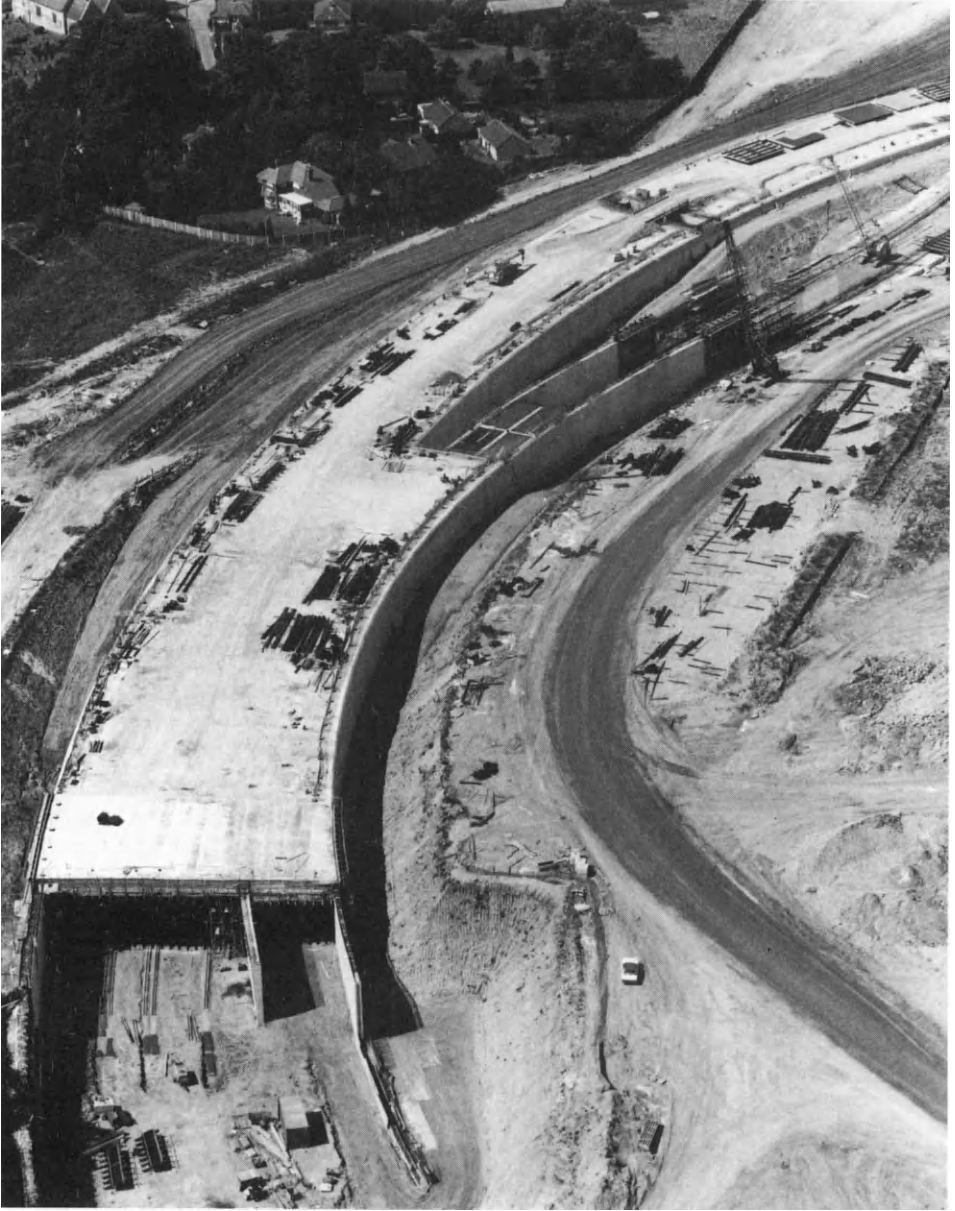
Figure 6.4 Terminal loop cut and cover tunnels, Channel Tunnel, UK. (Note secant pile walls in the left foreground and tapered intermediate wall)
