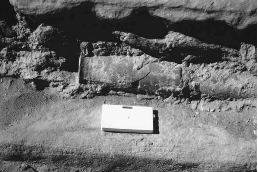
Figure 2.1.10. Nabataean thin wall short segment piping elements in the Great Temple forecourt (15 cm reference plate).
