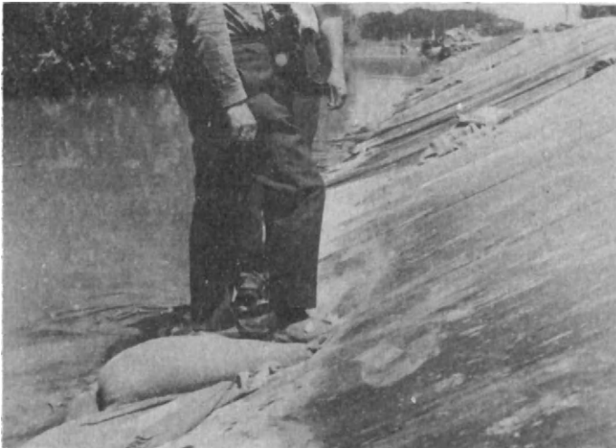
Fig. 5.21. Watertight plastic foil in the slope of a dam.
