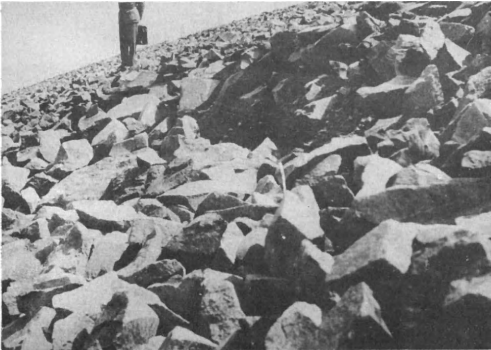
Fig. 3.16. Rip-rap failure of a dam.
