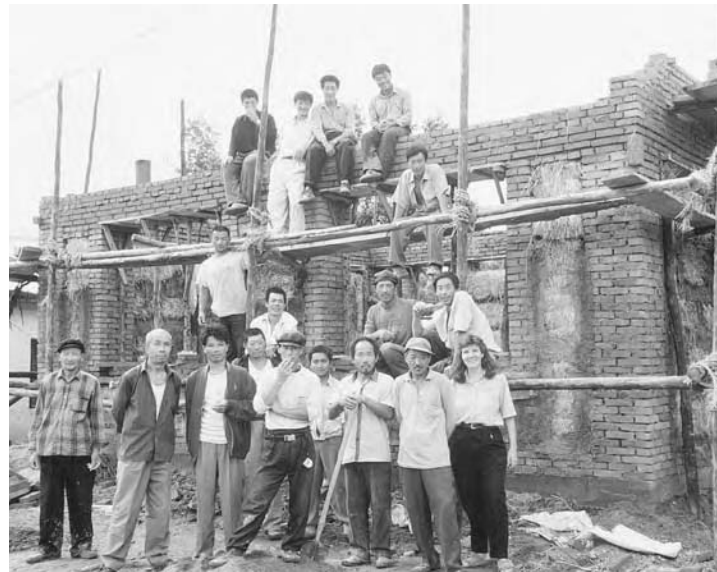
App-3: Kelly Lerner and Chinese builders in front of one of the projects built in China under the auspices of the Adventist Development and Relief Agency.
