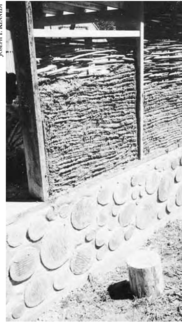
7-3: Wattle and daub uses small-diameter wood plastered with earth or lime plaster. It is an excellent infill system for moderate and benign climates.
