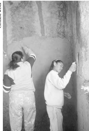
1-12: Caption: Local women plaster the interior of a new straw bale home in Anapra, Mexico.
