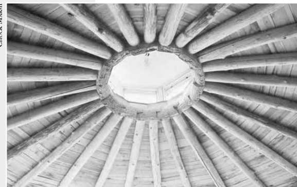
7-21: This example of round poles used to create an octagonal roof structure demonstrates the beauty of this locally available material. Using round poles in some situations, however, may demand a high level of craftsmanship for good structural connections and esthetics.
