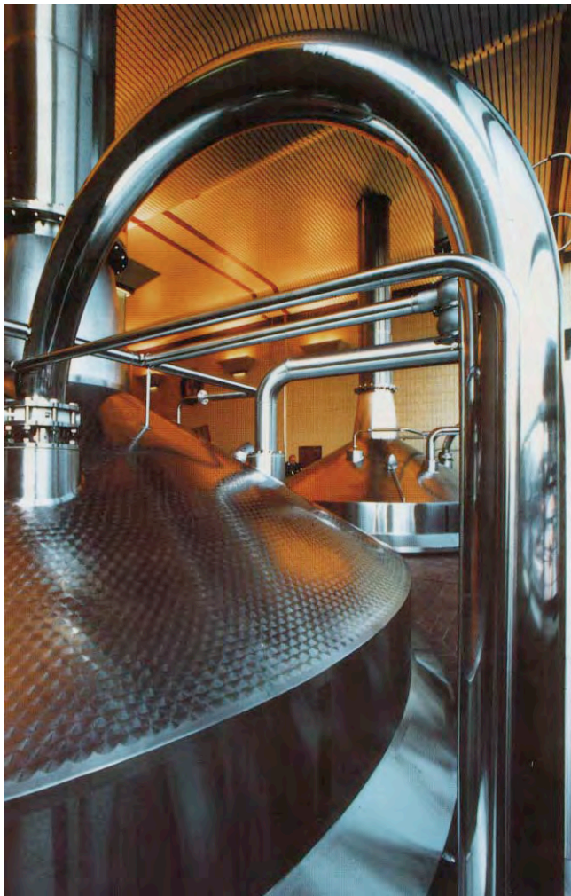
Plate 106 Metals Used in the Food Industry Stainless steel fermentation vessels and associated pipework in a modern brewery. (Courtesy of Courage Ltd and British Steel plc.)
