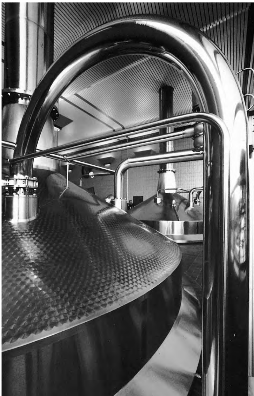
Figure 3 (see color plate 106) Stainless steel fermentation vessels and associated pipework in a modern brewery. (Courtesy of Courage Ltd and British Steel plc.)
