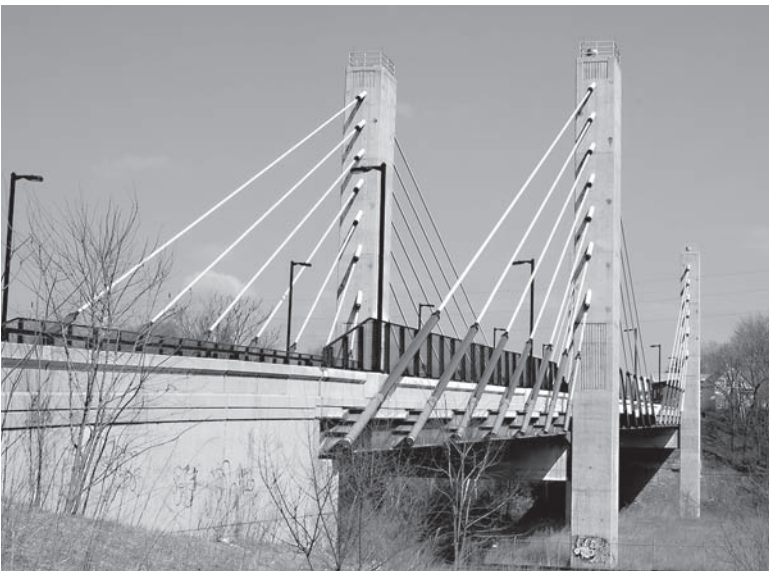
Figure 4. Arthur DiTommaso Bridge, also known as the Fifth Street Bridge, in Fitchburg, Massachusetts.
