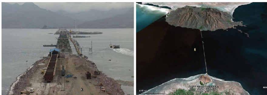
Fig. 2 Shahid Kalantari causeway across Urumia Lake; left side : construction in early stages; right side : causeway divides the lake into two separate parts (tebyan.net 2009)
