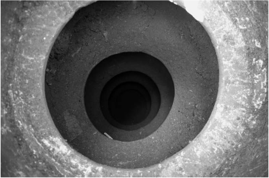
FIGURE 7.1. Well lining constructed of dolia with bottoms removed at Piammiano. Photo: JTP.
