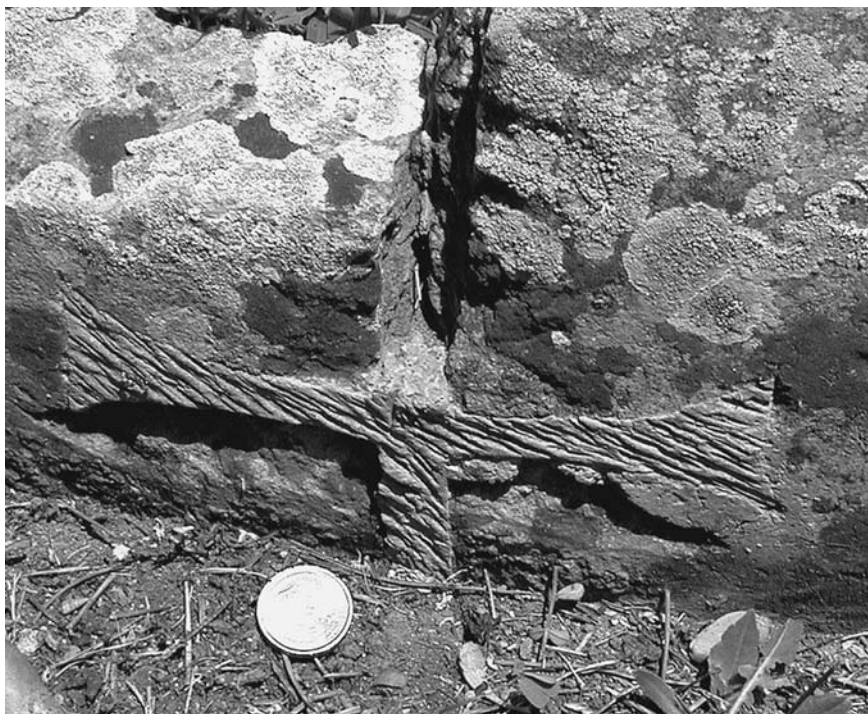
FIGURE 8.4. Detail of mortise and tenon technique repair to dolium defossum at Caseggiato dei Doli. Double-dovetail tenon and fill, with fill above tenon stripped away, showing reworking of crack into V-shaped channel. One Euro coin (diameter 2.4 cm) used to indicate scale. Photo JTP.
