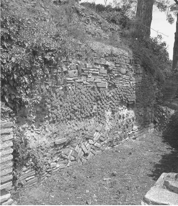
FIGURE 9.1. Opus caementicium wall with facing consisting in part of recycled pieces of pottery at Domus di Giove Fulminatore at Ostia. Photo: JTP.
