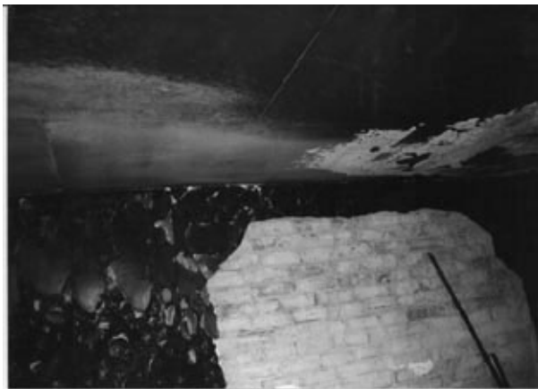
Figure 1 Plaster spalled from a wall as a result of cooling by fire fighting jets. The direction of the spray can be seen from displaced soot on the ceiling.
