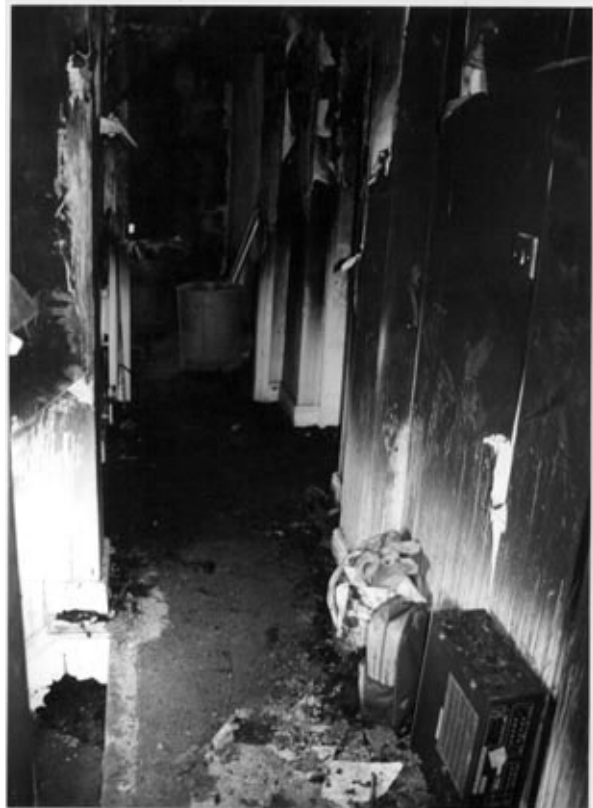
Figure 3 Typical smoke-logging in a passageway. Hot, buoyant smoke produces staining at a high level.
