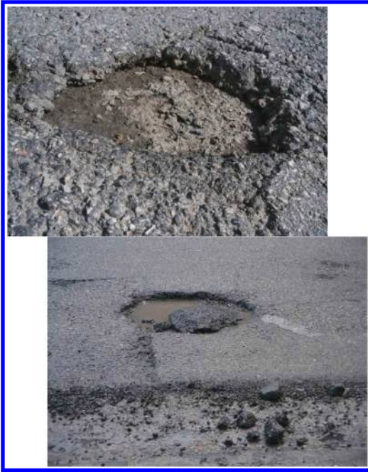
Figure 1. Examples of potholes.
