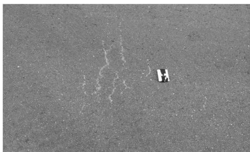
Figure 1. (b) The same crack in March 31, 2014.
