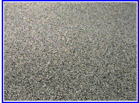
Figure 9. Surface details between junction 5 and 6, westbound 2014).
