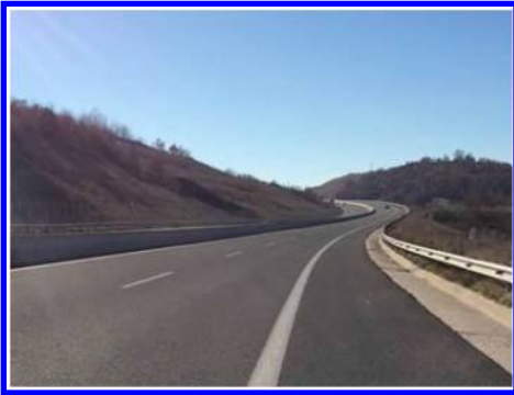
Figure 12. Pavement after eight years in service between junction 7 and 8, westbound (year 2014).
