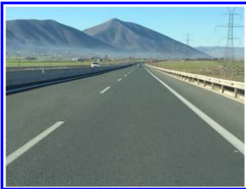
Figure 8. Pavement after eight years in service between junction 5 and 6, westbound (year 2014).
