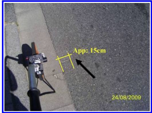
Figure 3. Lateral crack at the edge.
