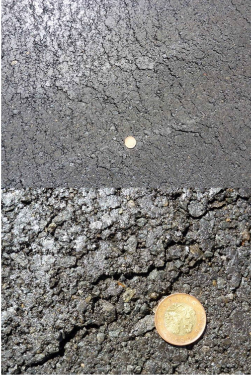
Figure 4. Compaction of cold emulsified asphalt mix layer/Appearance of compacted layer (transverse surface cracks which should be “smoothed” by suitable roller).
