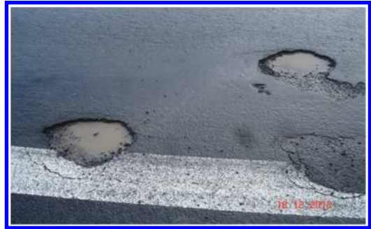
Figure 5. Pot holes appeared at a bridge deck in Egnatia motorway.
