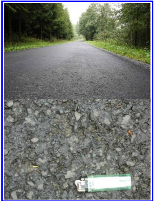
Figure 5. Sub-section No. 1 – material loss in the wearing course.
