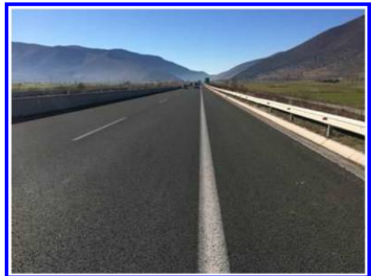
Figure 10. Pavement after eight years in service between junction 6 and 7, westbound (year 2014).
