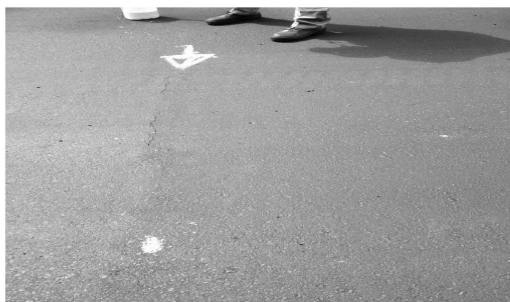
Figure 1. (a) Crack that appeared in March 1, 2013.
