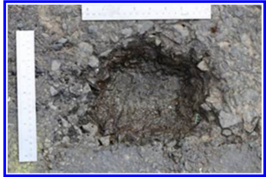
Figure 6. Real in-situ pothole with steel rules for control purposes.
