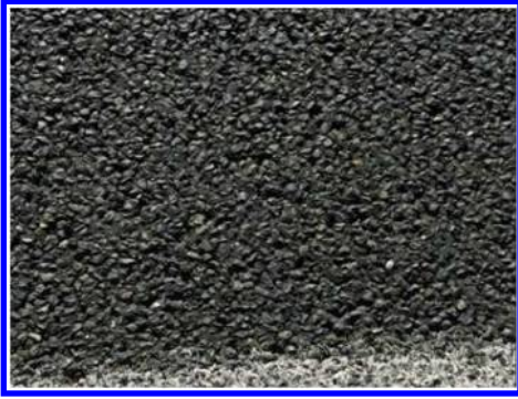
Figure 11. Surface details between junction 6 and 7, westbound 2014).
