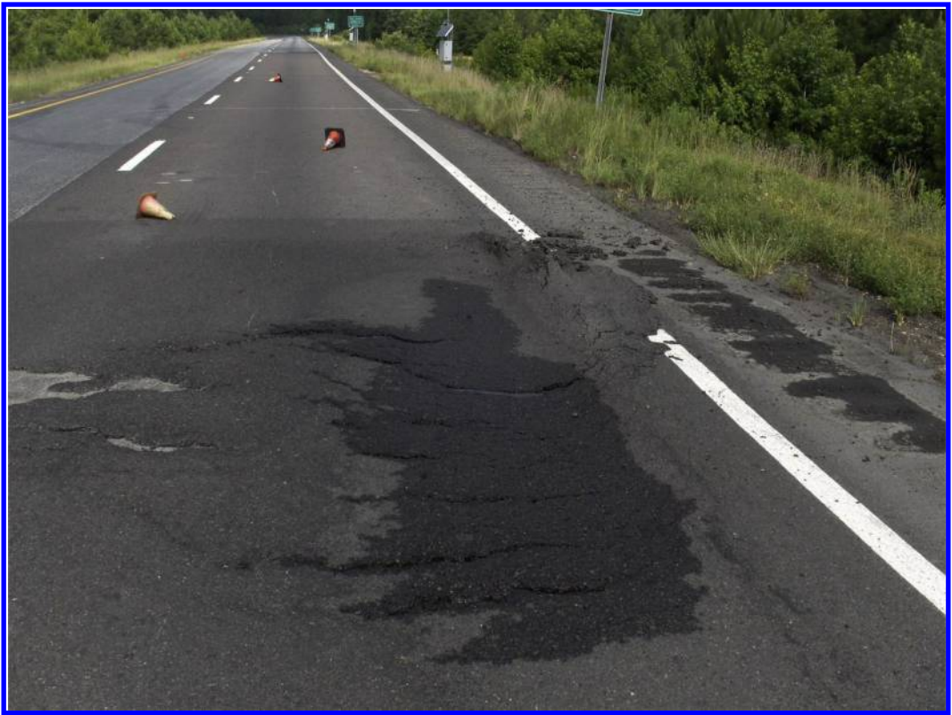
Figure 9. N8 pavement failure after conventional mill and inlay.
