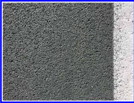
Figure 13. Surface details between junction 7 and 8, westbound 2014).
