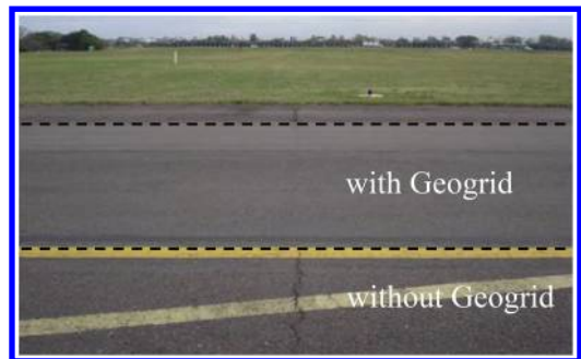
Figure 6. Joints of the concrete slabs reflect in the area where no reinforcement was used.
