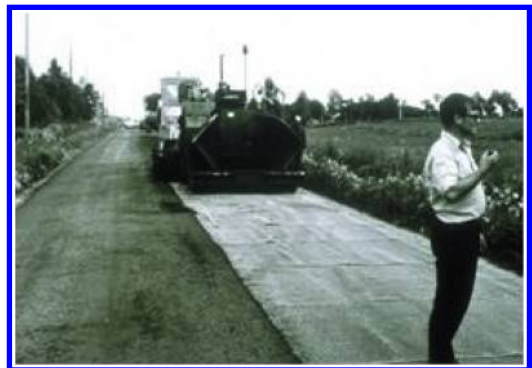
Figure 1. One of the first attempts to use a geogrid in asphalt pavement at the early 1970s.
