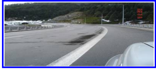
Figure 4. Pot holes and raveling appeared at a downgrade bridge deck in Egnatia motorway.
