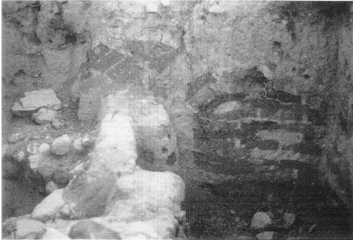
Figure 4.10. Cross-section of a mud-brick wall at Tel Hazor north of the Sea of Galilee and along the major strike-slip fault of the Dead Sea–Jordan rift—destroyed probably by an ancient earthquake.
