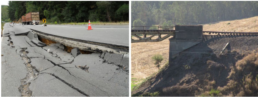
Fig. 1.35 Ground failure in a highway ( left panel ) and extensive settlement in a railroad bridge abutment ( right panel ) during the 2010 Maule, Chile earthquake (EERI Earthquake Photo Gallery)
