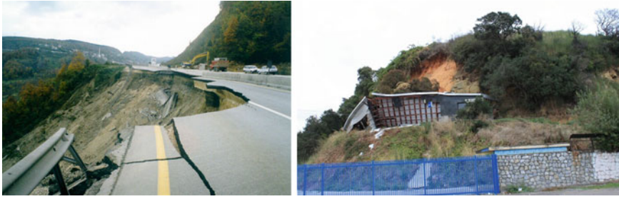
Fig. 1.38 Landslide at a highway embankment during the 1999 Düzce earthquake ( left panel ) and landslide directly above structure during the 2010 Maule, Chile earthquake ( right panel , EERI Earthquake Photo Gallery)
