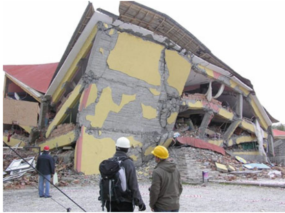
Fig. 7.32 A squat shear wall failed during the 2011 Van Earthquake
