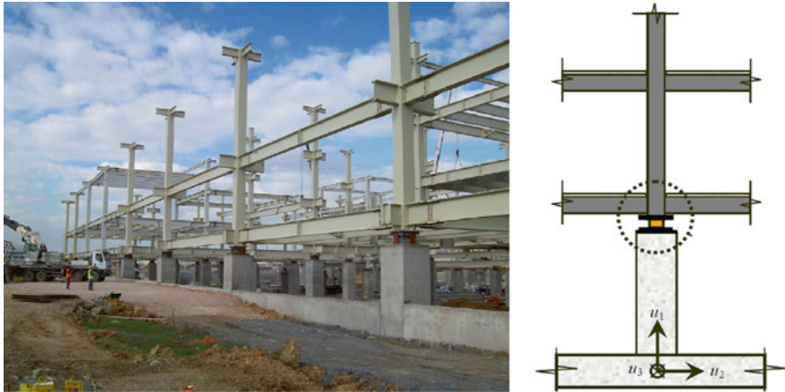
Fig. 5.17 Base isolation interface between concrete basement and steel upper structure of a building
