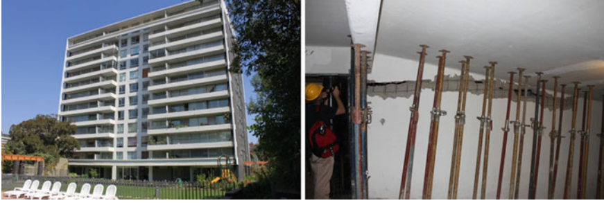
Fig. 7.30 Shear wall damage at the ground story of a modern concrete building during the 2010 Chile earthquake (M 8.8)
