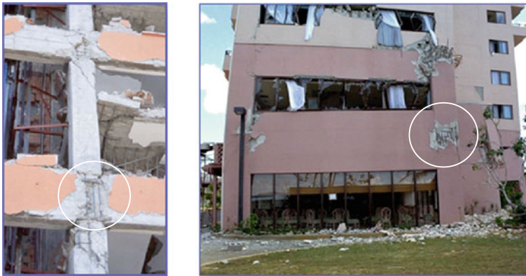
Fig. 7.23 Joint failures observed in non-ductile reinforced concrete buildings due to strong ground shaking (from Moehle et al. 2004)
