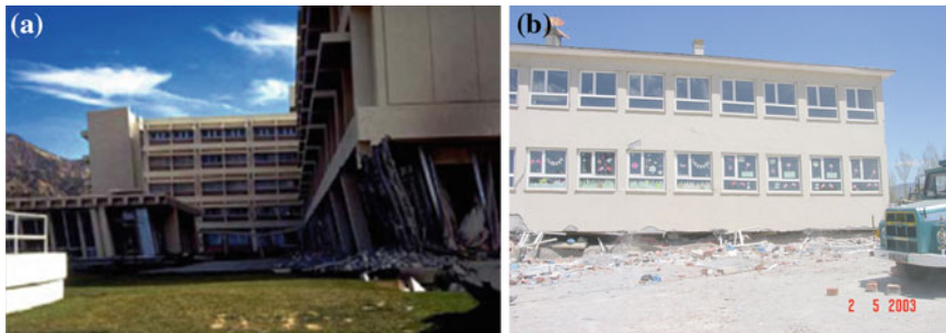
Fig. 7.15 Soft story collapses from a 1971 San Fernando Earthquake, USA on the left, b 2003 Bingöl earthquake, Turkey on the right
