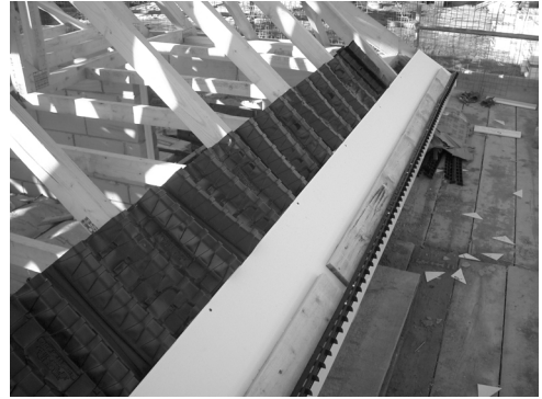
B Ventilator installed over rafters at eaves.
