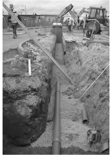
B The laser can be used to obtain a level for the pipe bedding, the drainage is placed onto the bedding and positioned to correct fall
