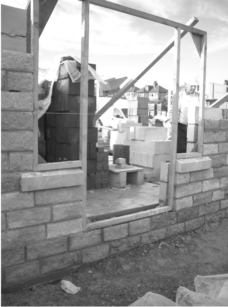
A Temporary window and door template, used to ensure that the wall opening is built to the correct size to receive the window and doorframe.
