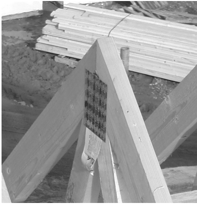
A Gang nail plate holds members of the truss in position
