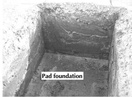
B This pad foundation has been excavated down to good loadbearing strata. The bottom of the foundation is clean and ready for inspection by the building control officer.
