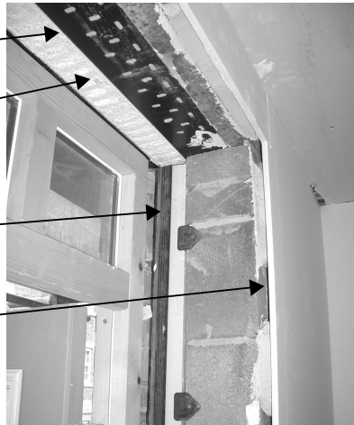
C Underside of lintel can be seen, plaster board will be used to cover the exposed lintel
