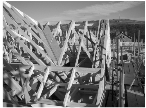
B Cavity sock seals the top of the cavity at gable end
