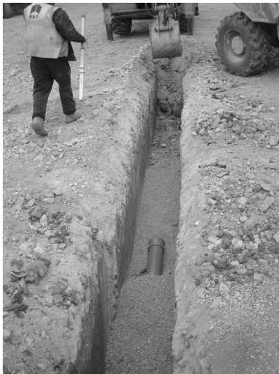
C Once the pipe is correctly positioned pipe bedding covers the whole pipe
