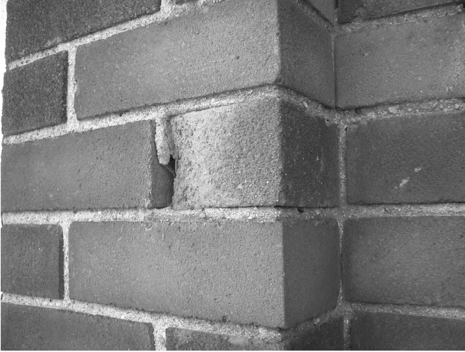
Photograph 5.1 Face of brickwork removed by frost attack
