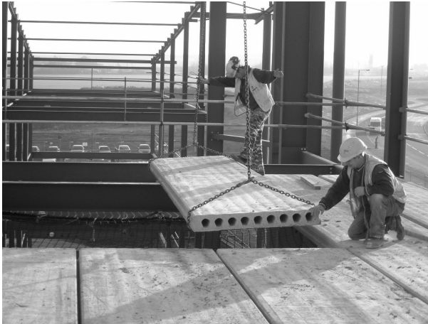
B Each beam is hoisted into position and placed on the supporting walls or beams
