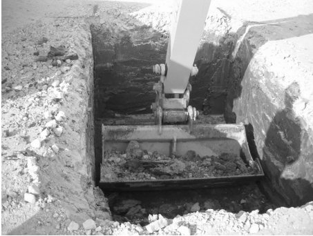
A The foundation is marked out and excavated to the correct level. The machine operator attempts to keep the sides of the excavation as true and square as possible.
