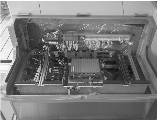
Figure 5: Photo[4]VORS Equipment Assembly on in Compartment
