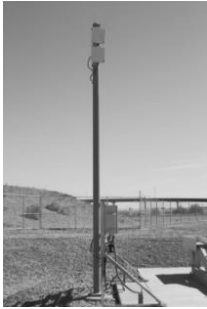
Figure 1: Photo[1] Access point on free standing pole.
