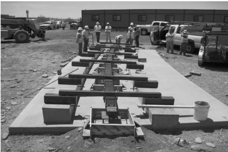
Figure 7. Guideway Cross Section Means and Methods Development (Source: BT Construction/Installation of Phoenix Sky Train)
