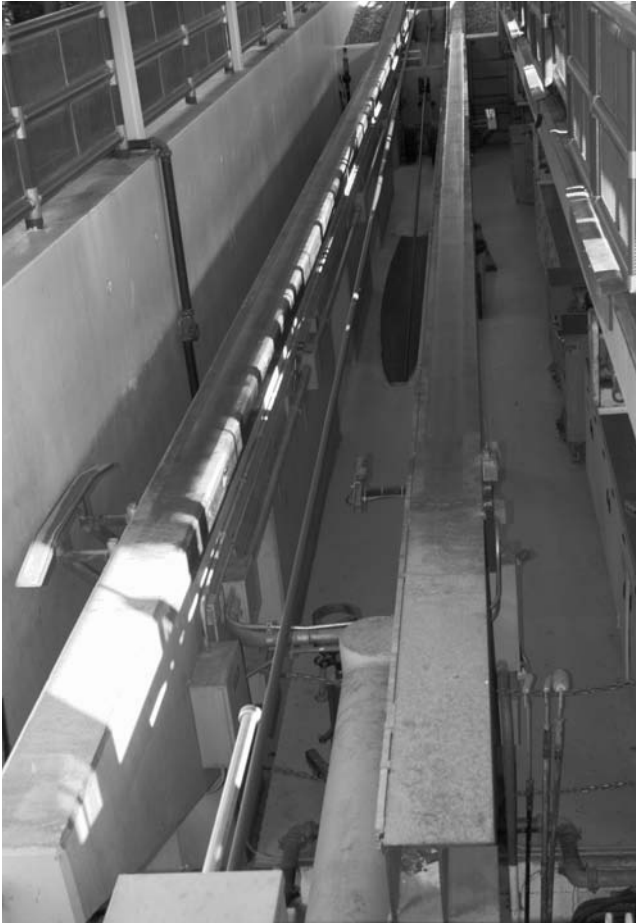
Figure 2. Mirage/TI APM Guideway.
