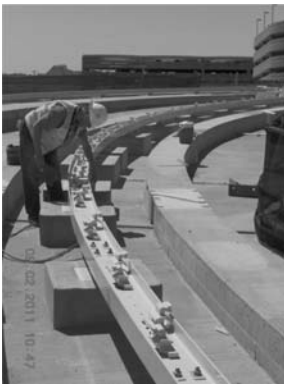
Figure 21: Power Rail Brackets
