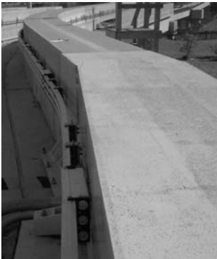
Image 23: 400A conductors installed at the point of a multi-position switch, Conductix, Inc.
