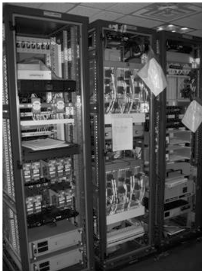
Figure 7: Wayside Cabinets in Factory Acceptance Test - Bombardier
