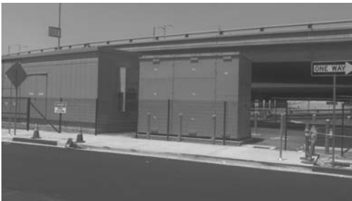
Figure 2-2 - Typical TPSS Courtesy of HART
