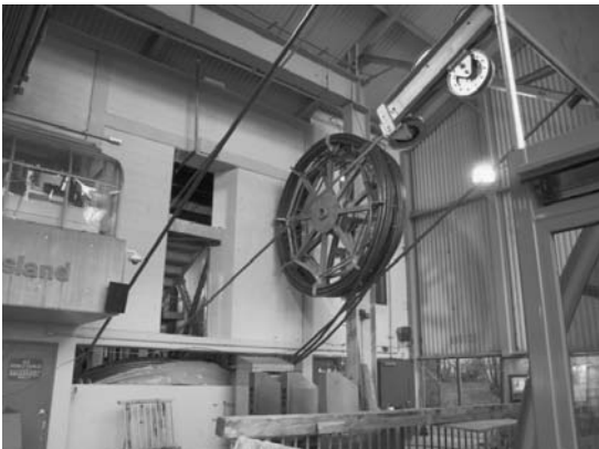
Picture 6 – New Machine Room Enclosure (ESG)
