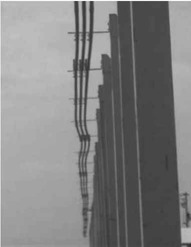
Image 19: Poor expansion management can cause conductor snaking and loss of collector contact, Conductix Inc.
