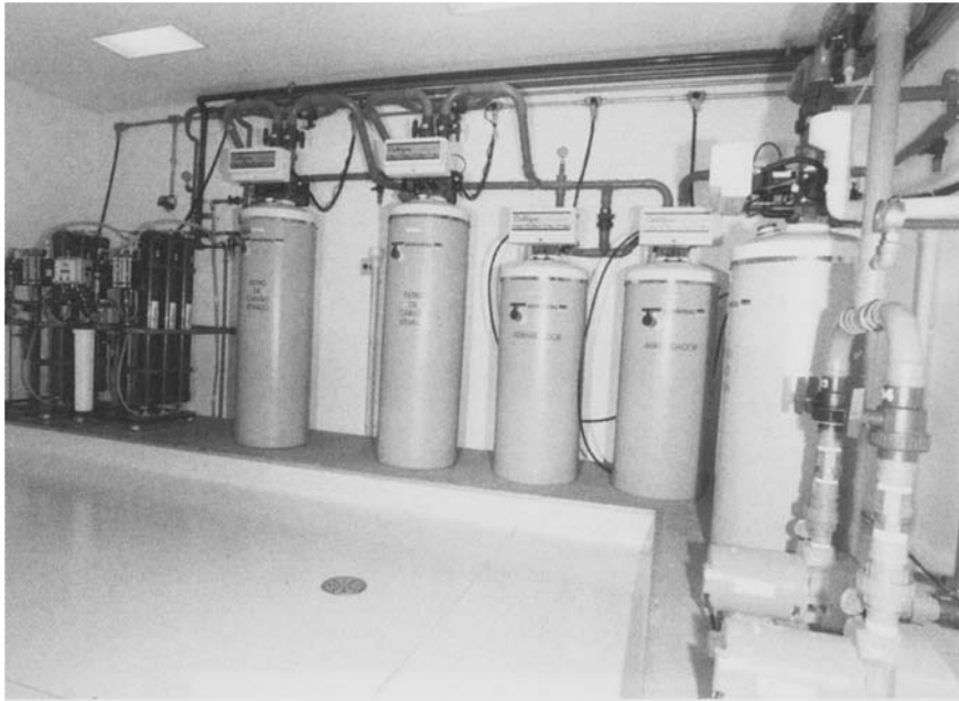
Figure 1. Water treatment system in a Brazilian private hospital. From right to left are seen one sand filter, two softeners (ion-exchange filters), two charcoal (carbon) filters, and a set of reverse-osmosis membranes.
