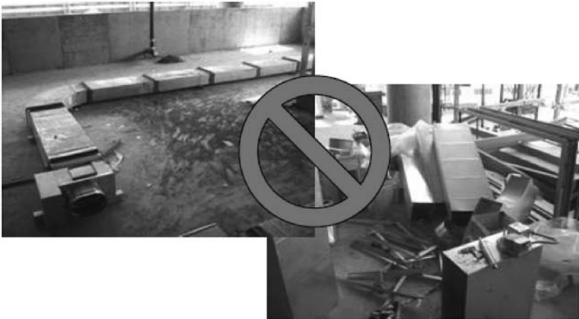
Figure 6-11 Bad construction IAQ management.
