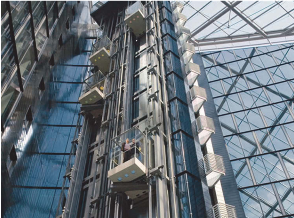
Figure 11.4 A multideck ThyssenKrupp Twin elevator system.
