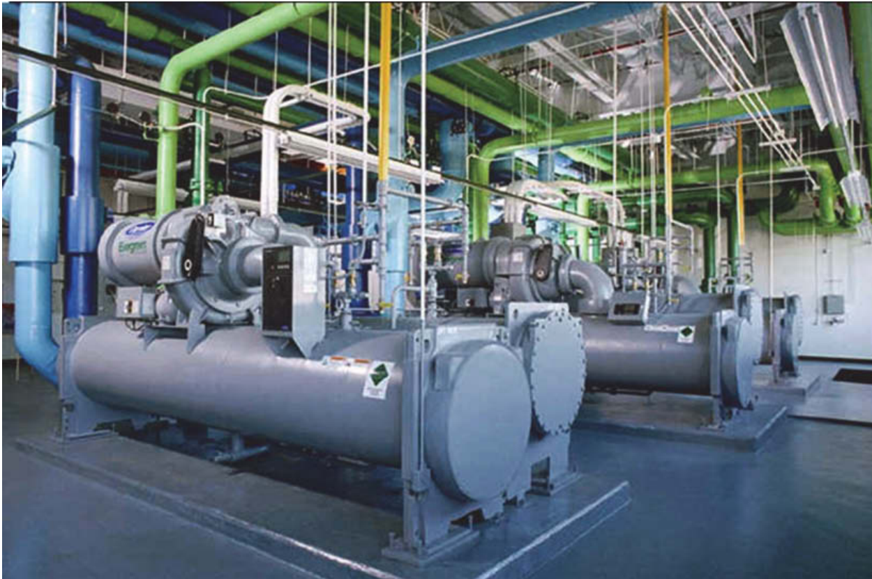
Figure 8.5 A typical basement plant room for multiple chillers.
