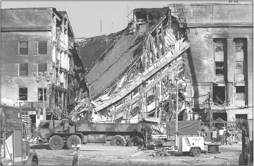
Section of the Pentagon building struck by the hijacked airliner. (Department of Defense, Still Media Records Center)
