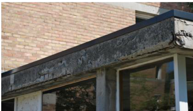
Figure 3.52 Degraded concrete due to steel bar corrosion.
