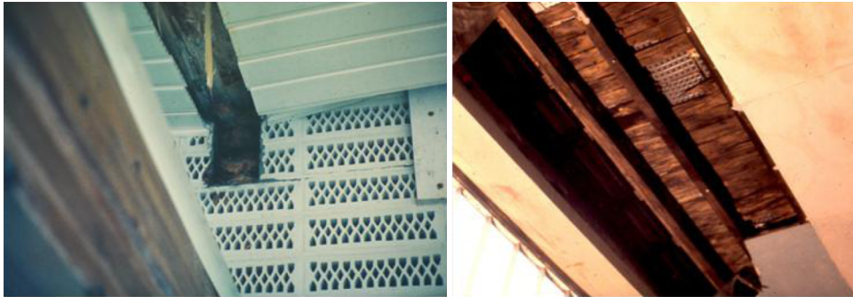
Figure 3.42 Natatorium. Left collapsed roof beam, right collapsed roof deck, both due to long-lasting interstitial condensation.
