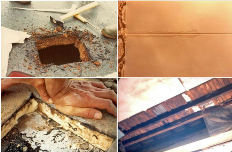
Figure 4.25 Damage caused by interstitial condensation.
