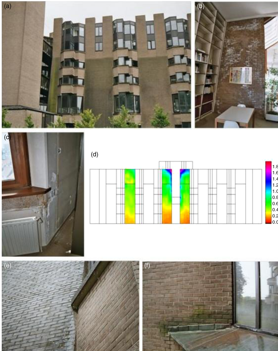
Figure 4.30 (a) The building, (b) moisture spots, (c) leakage along window sills, (d) catch ratio, (e) run-off, (f) no upward sill folds.
