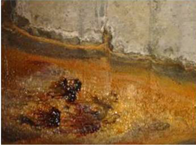
Figure 4.19 Natatorium, leaking swimming pool wall.
