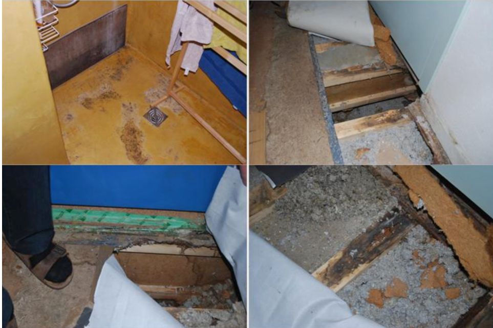
Figure 4.21 Damage caused by a leaky hot water pipe.
