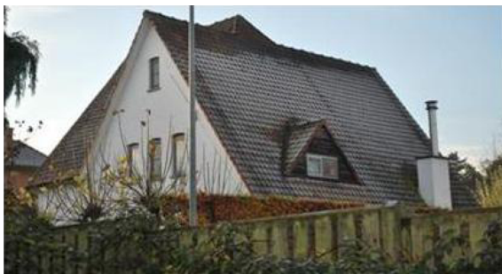
Figure 1.9 Rime formation on a well-insulated pitched roof due to under-cooling.
