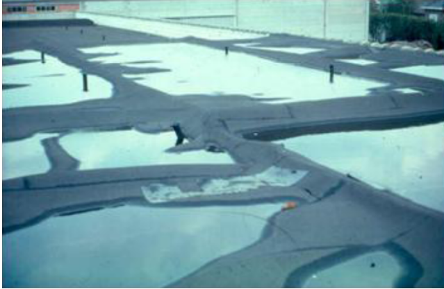
Figure 3.44 Low-sloped roof above a timber kiln, irreversible deformation of PUR.
