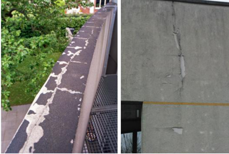
Figure 3.46 Cracks degrade appearance.
