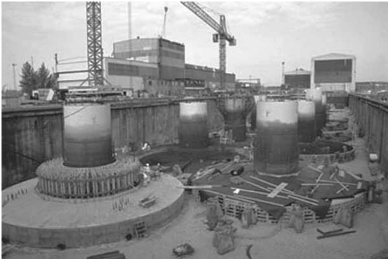
16.26 Construction of gravity based foundations for the offshore wind farm Middelgrunden in a dry dock (© Middelgrunden Wind Turbine Cooperative).
