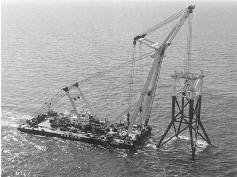
16.25 Positioning and sinking of a jacket using a floating crane (© F + Z Baugesellschaft mbH, Hamburg).
