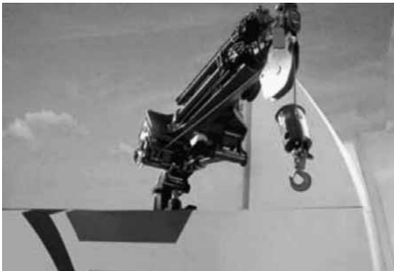
18.2 Examples of internal cranes in the Siemens 3.6 (top) and Repower 5 M (bottom) turbines.
