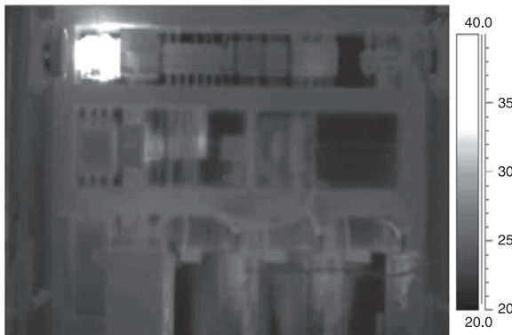
11.6 Thermo image of an electrical cabinet.
