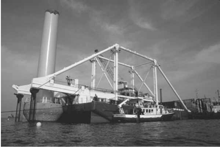
16.27 Transport of a gravity based foundation to the location of the offshore wind farm Middelgrunden (© Middelgrunden Wind Turbine Cooperative).
