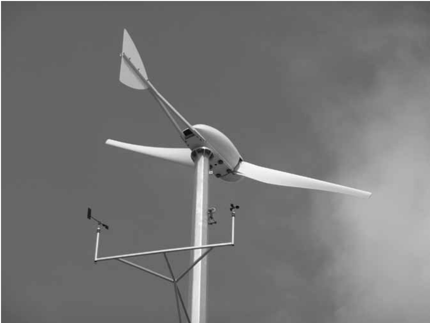
13.8 The Aerogenesis 5 kW wind turbine with cup anemometer and wind vane.
