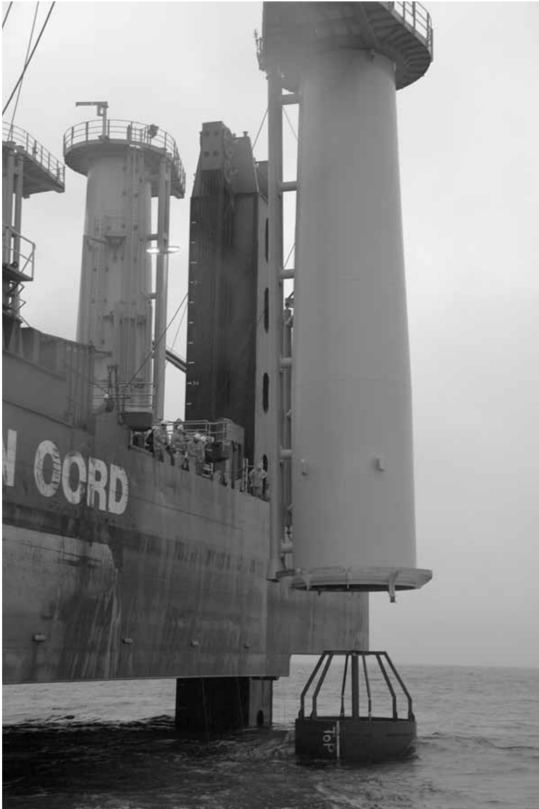
16.24 Transition piece installed by Van Oord at Q7, Prinses Amalia WP (© Van Oord Dredging & Marine Contractors).
