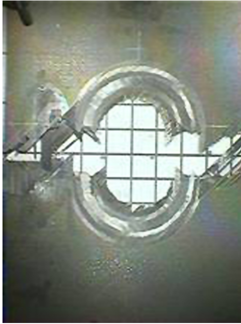
Figure 26.13 The front of scarfed panel 419T after failure.
