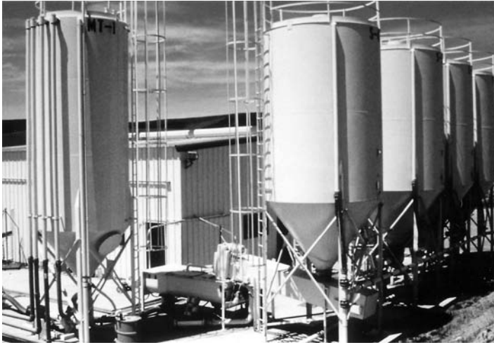
FIGURE 7.15 Solidification process. Lime and fly ash storage and dispensing.
