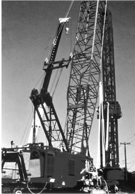
FIGURE 11.14 Deep soil mixing equipment used in situ solidification. (From Geo-Con Incorporated, 4075 Monroeville Blvd., Suite 400, Monroeville, PA 15146. With permission.)
