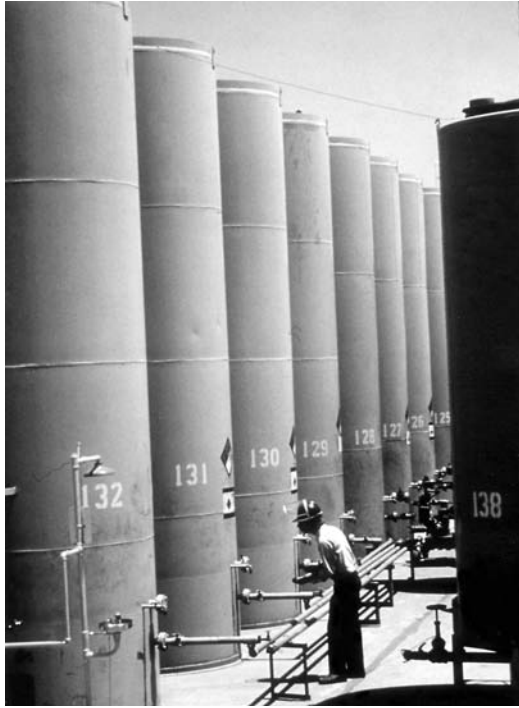
FIGURE 7.25 Hazardous waste storage tanks with secondary containment.
