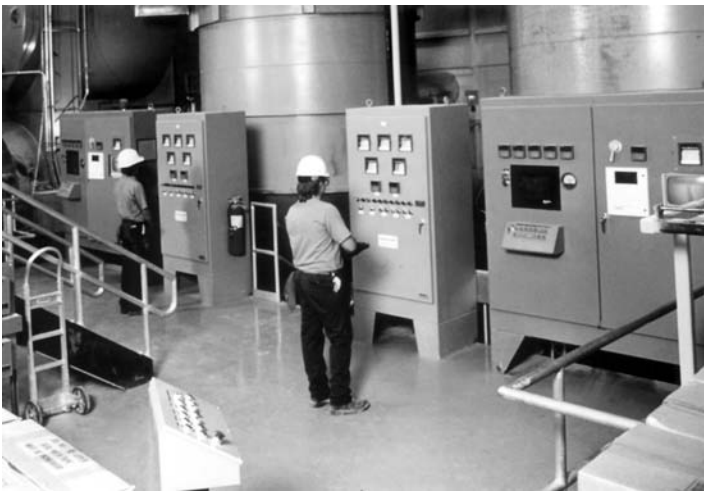
FIGURE 12.11 Combustion controls for an infectious waste incinerator.
