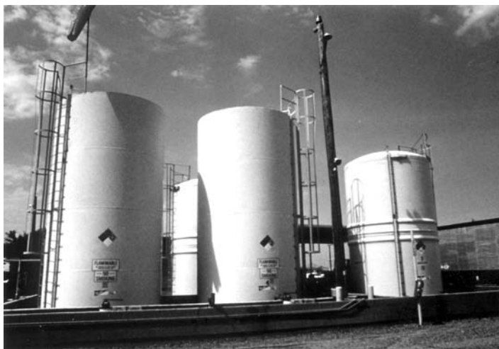
FIGURE 7.24 Hazardous waste storage tanks with secondary containment.
