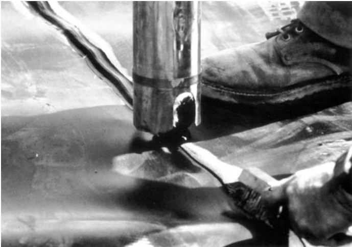
FIGURE 7.29 Land disposal liner sections being welded. (From GSE Lining Technology, Inc., 19103 Gundle Rd, Houston, TX 77073. With permission.)
