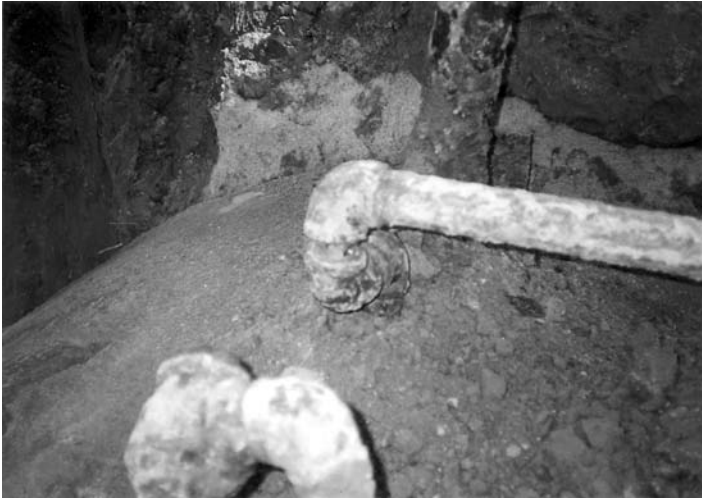
FIGURE 14.4 Typical corroded piping at an underground storage tank replacement site. Note hole in pipe nipple between elbows. (From Environmental Technology, Inc., 2541 E. University, Phoenix, AZ. With permission.)
