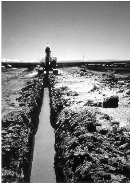
FIGURE 11.2 Cement-bentonite cut-off wall. (From Geo-Con Incorporated, 4075 Monroeville Blvd., Suite 400, Monroeville, PA 15146. With permission.)
