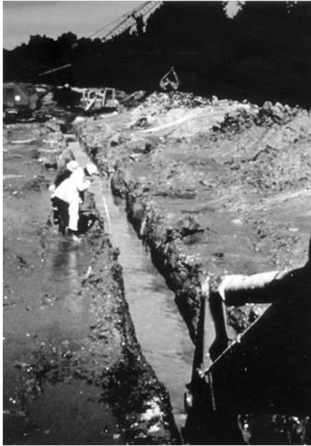
FIGURE 11.1 Soil-bentonite slurry wall construction. (From Geo-Con Incorporated, 4075 Monroeville Blvd., Suite 400, Monroeville, PA 15146. With permission.)
