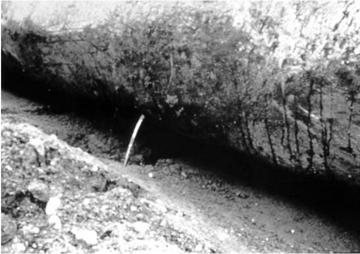
FIGURE 14.3 Typical pinhole leak caused by galvanic activity. (From U.S. Environmental Protection Agency.)
