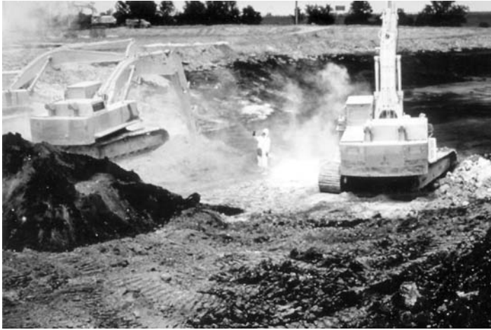
FIGURE 11.13 Solidification by in situ mixing using backhoes. (From Geo-Con Incorporated, 4075 Monroeville Blvd., Suite 400, Monroeville, PA 15146. With permission.)
