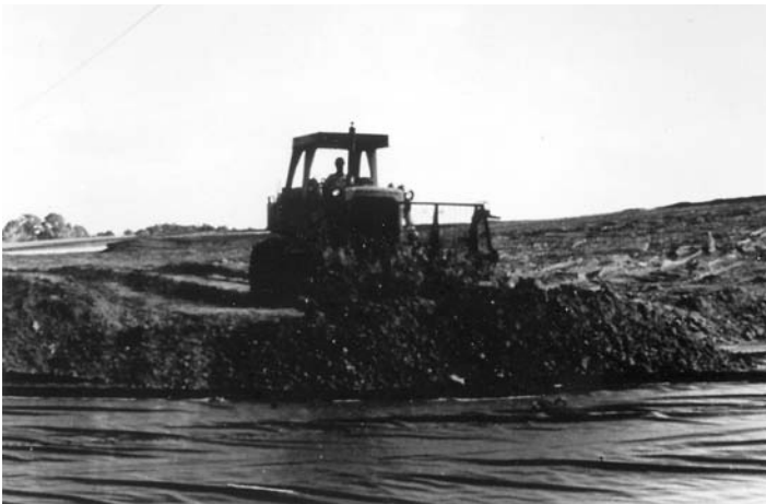
FIGURE 7.31 Liner bedding for protection from puncture. (From GSE Lining Technology, Inc., 19103 Gundle Rd, Houston, TX 77073. With permission.)
