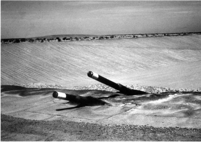
FIGURE 7.32 Secure landfill leachate detection and monitoring access. (Courtesy of Safety-Kleen Corporation.)
