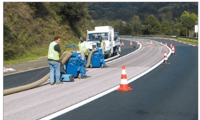
FIGURE 6-27: Asphalt pavement can be abraded with shot blasting to remove the black asphalt from the surface. This process exposes the aggregate in the asphalt pavement. If it is a light-colored aggregate, the surface will be lightened and reflect more solar radiation, reducing the pavement’s contribution to the urban heat island effect.
