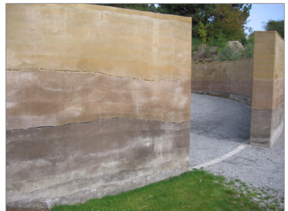
FIGURE 6-31: Constructed and rammed in lifts, rammed earth walls have variations in color among the lifts due to variations in soil color.
