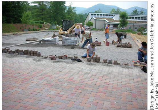
FIGURE 3-31: Permeable unit paving installed over a washed gravel dry well capable of retaining the 10-year storm event at the North Carolina Arboretum.
