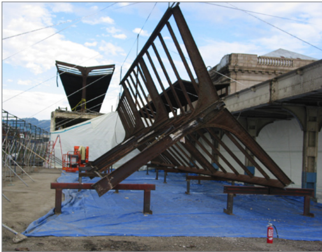
FIGURE 6-6: Miller Company Landscape Architects “mined” steel canopy structures from a nearby defunct train station and repurposed them for reuse at the 14th Street Pocket Park in Oakland California.
