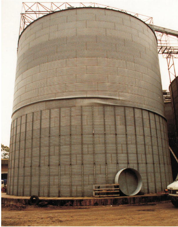
14.15 Failure by corrugation collapse.
