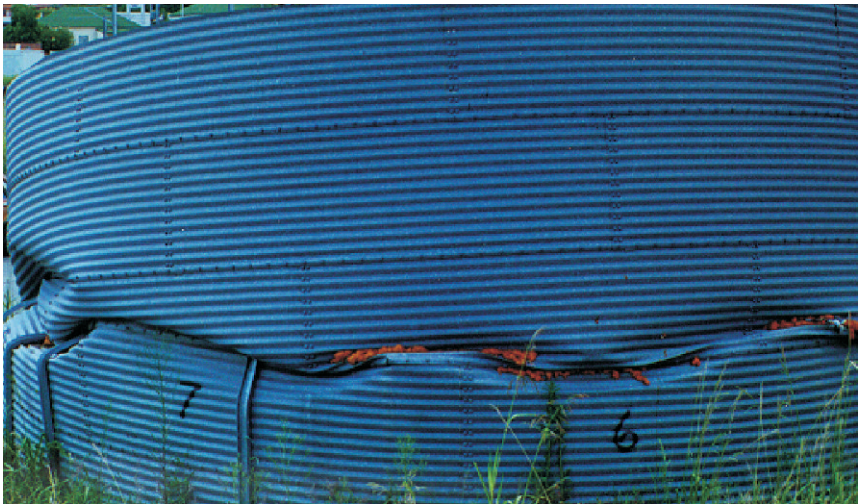
14.16 Corrugation collapse at end of stiffeners.
