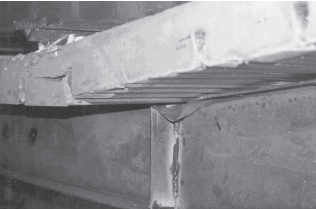
8.11 Local buckling of a composite steel–concrete beam (Uy and Sloane, 1998).
