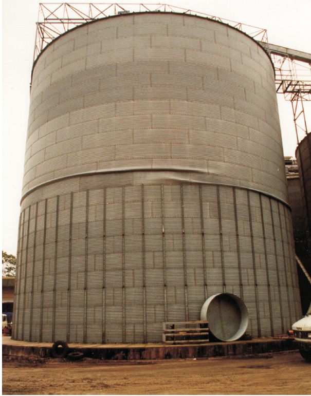
14.15 Failure by corrugation collapse.
