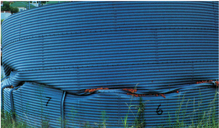
14.16 Corrugation collapse at end of stiffeners.
