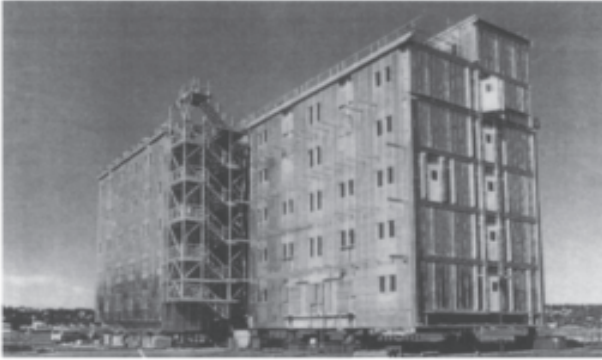
One of the aluminium accommodation modules for the Saga oil-field in the North Sea, before float-out. Welded up from 0.5 m wide extrusions by Leirvik Sveis on Stord Island, Norway, 1990.
