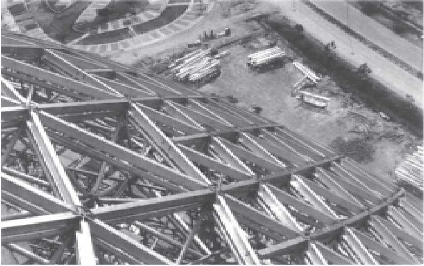
Aluminium structure for the 51m diameter dome on the Selangor State mosque, at Shah' Alam, Malaysia, 1987. Built by BACO Contracts, using their 'Triodetic' system.
