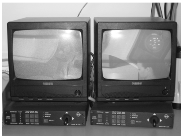
FIGURE 14.7. A remote monitor bank.
