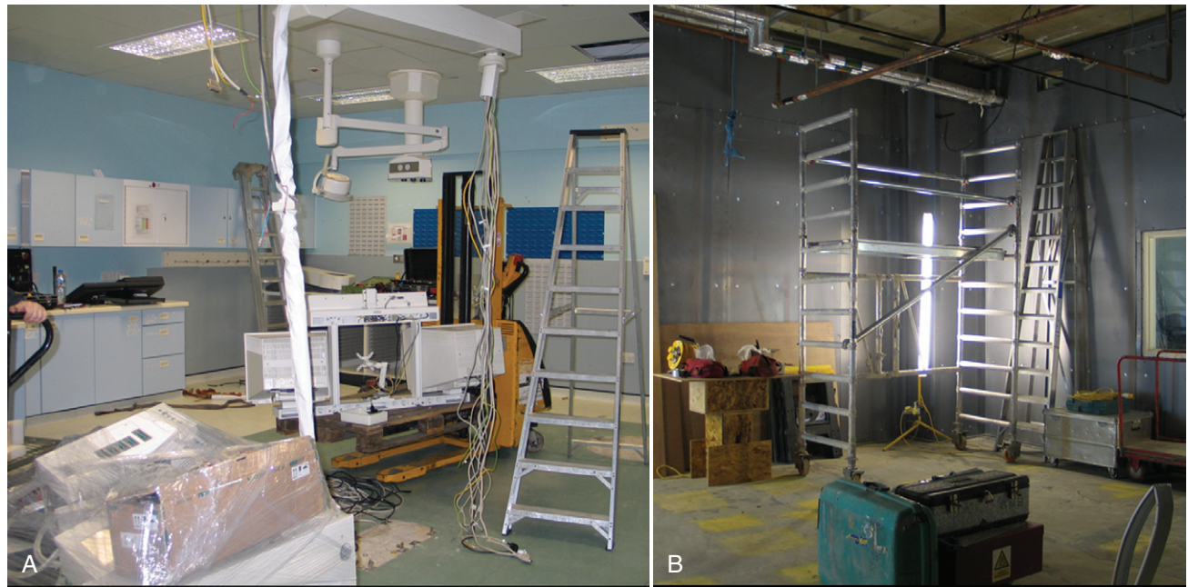
FIGURE 21-1 Retrofit of a conventional catheter laboratory. A , The old equipment is removed. B , The examination room's walls are fitted with special shielding.
