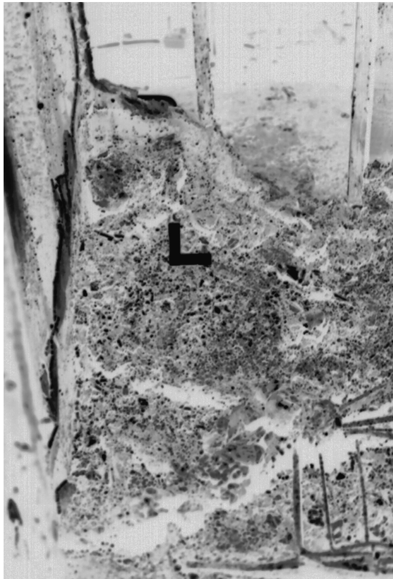
Figure 23.4 View of fire-damaged closet containing the remains of two young fire victims.
