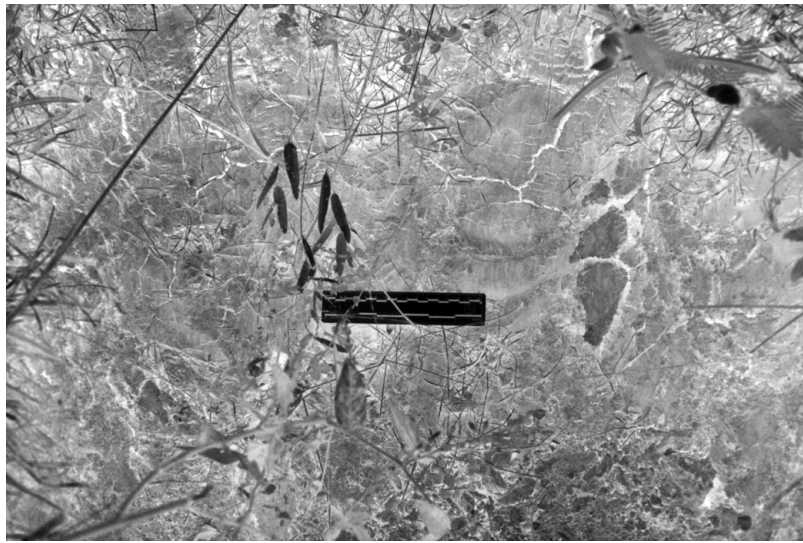
Figure 3.7 Subsurface desiccation and cracks formed in the walls of an open pit 1 day after excavation.
