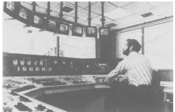
FIG. 5.51. Quarry process plant control room.
