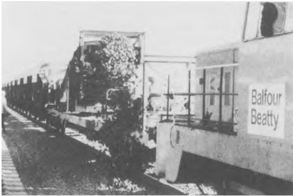
FIG. 12.1. Track ballast being delivered by self-discharging train (courtesy Balfour Beatty Railway Engineering Ltd).
