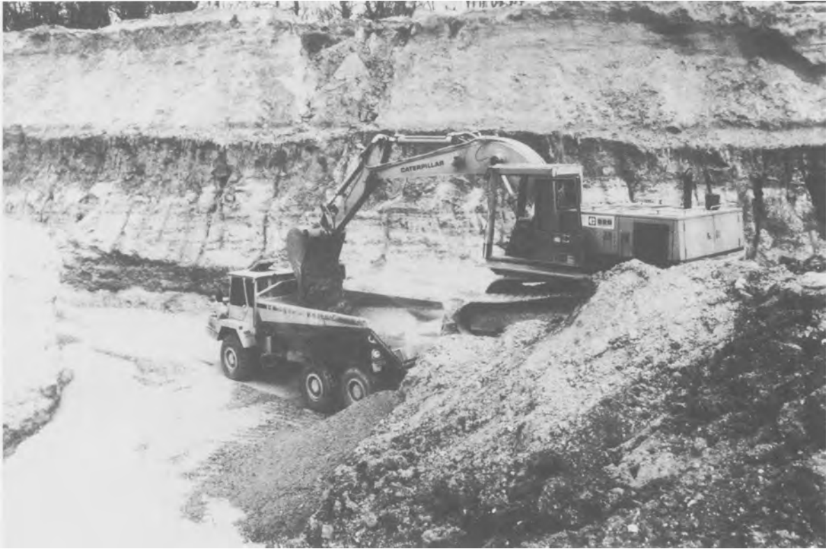
FIG. 4.4. Hydraulic back-hoe excavator and articulated dump truck used to remove overburden and excavate sand and gravel (courtesy of Redland Aggregates Ltd).
