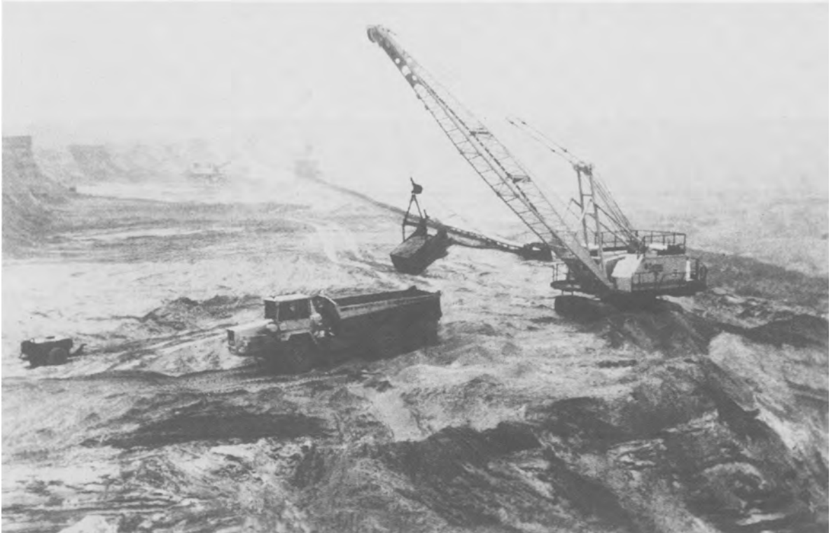
FIG. 4.20. Dragline excavator with ADT and field conveyor system (courtesy of RB (Lincoln) Ltd).
