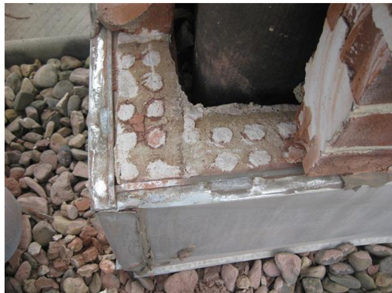
Fig. 13. Poorly installed roof interface flashing almost always leads to interior water leakage.
