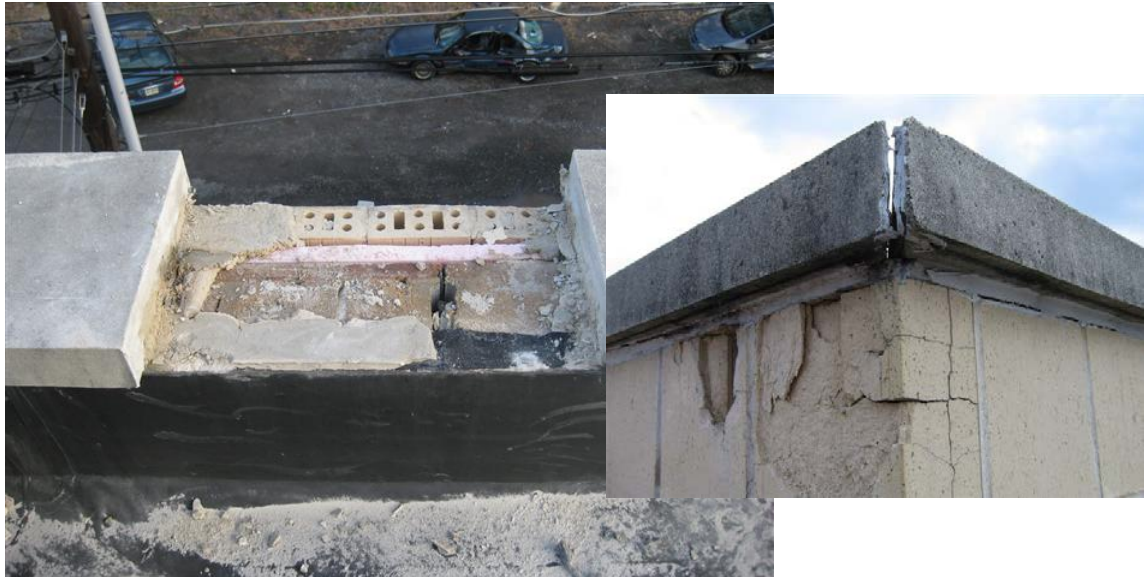
Fig. 4. The lack of through-wall flashing below the coping allowed substantial water infiltration into the parapet, causing significant deterioration of the brick veneer.
