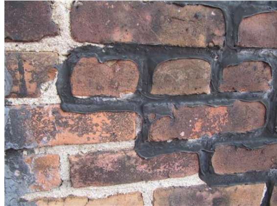
Fig. 17. Sealant application traps moisture within the masonry.
