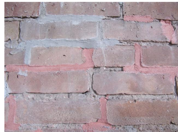
Fig. 9. Multiple generations of mortar joint repointing.
