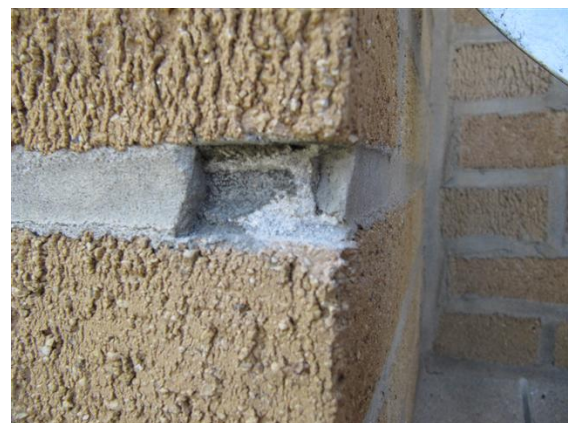
Fig. 12. Thinly applied mortar over existing mortar will result in poor performance.
