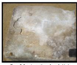
Figure 2: Sugaring on the surface of a block
