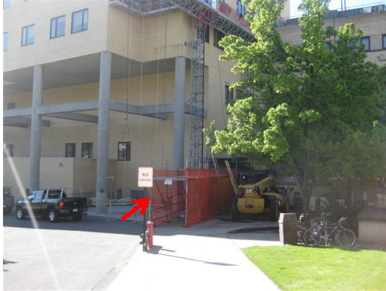
Fig. 12. Overhead protection allows continued use of the entrance while long-term restoration repairs are being completed.
