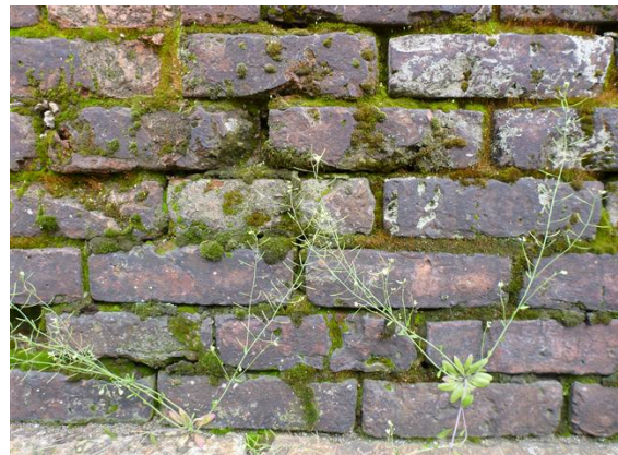
Fig. 3. Excessive plant growth contributing to mortar joint deterioration.
