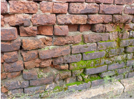
Fig. 4. Mortar joint erosion.
