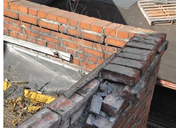
Fig. 5. Unstable masonry areas as a result of mortar joint bond loss.
