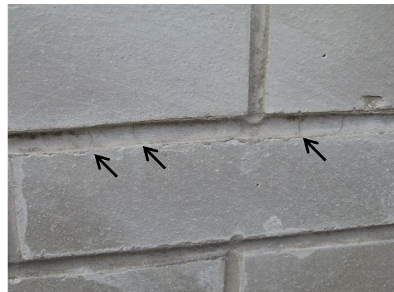
Fig. 11. Drying shrinkage cracks from too wet mortar.
