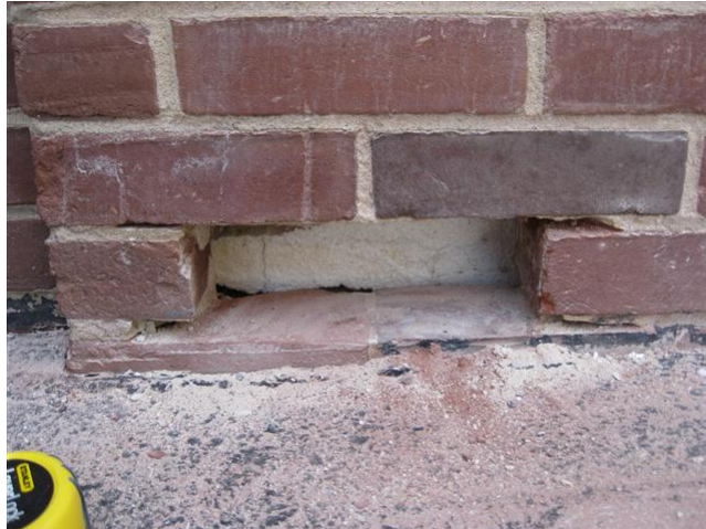
Fig. 14. Without through-wall flashing at the base of the building, water will remain in the wall system.
