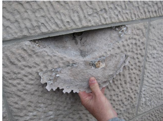
Fig. 5. A large limestone spall was removed by hand from the façade.
