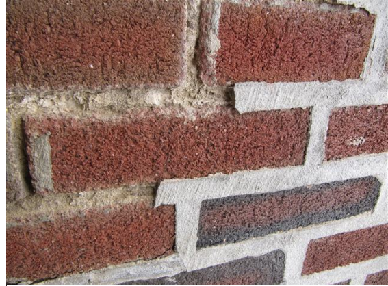
Fig. 13. Failure of grout installed over deteriorated mortar joints.
