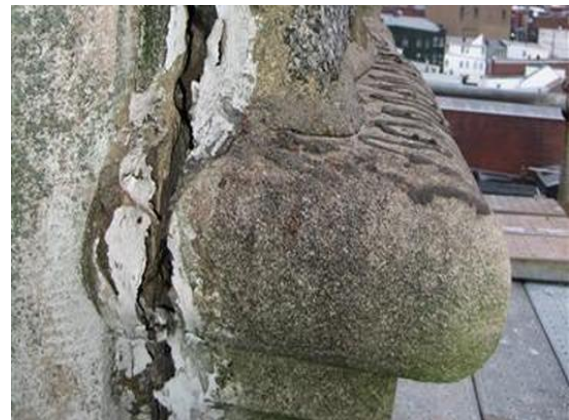
Fig. 6. Out of plane masonry displacement.
