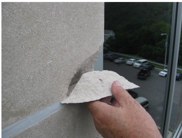
Fig. 6. Loose pieces can be removed whenever feasible as long as doing so will not contribute to additional deterioration of the façade.
