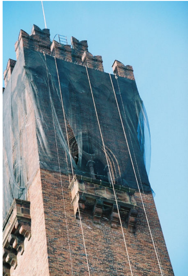
Fig. 9. Poorly installed netting done by personnel without the appropriate expertise.
