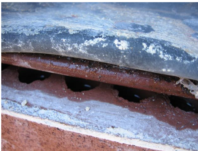
Fig. 1. Poorly installed flashing exposed the steel angle to excessive moisture and allowed water to collect into the cores of the brick below.
