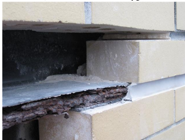
Fig. 7. Poor flashing details allowed water to continuously reach the steel angle, rapidly increasing the rate of corrosion of the steel.
