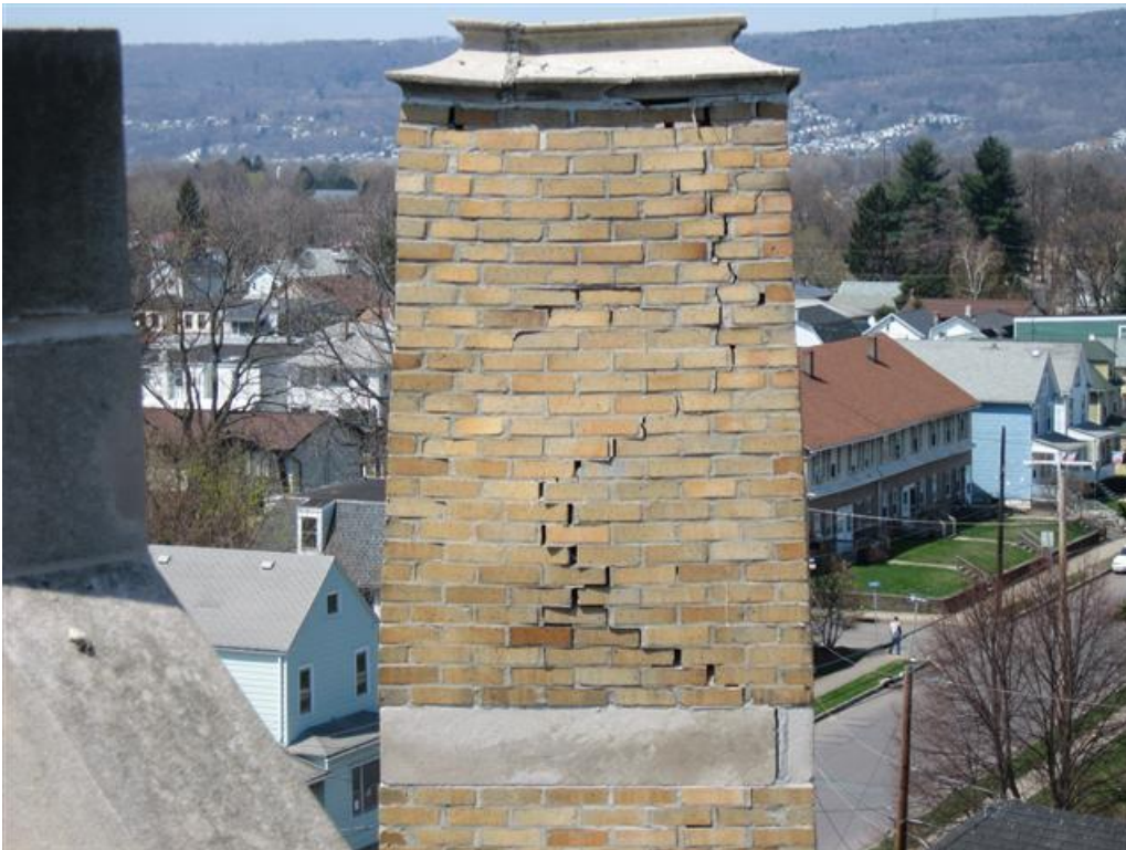
Fig. 1. Masonry chimney with severe displacement of the masonry has become an unsafe condition.
