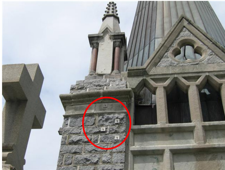
Fig. 7. Stainless steel anchors and plates support the masonry that was displacing away from the wall.
