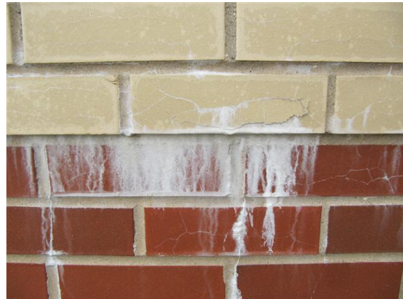
Fig. 2. Lime deposits on the masonry surface resulting from water infiltration.
