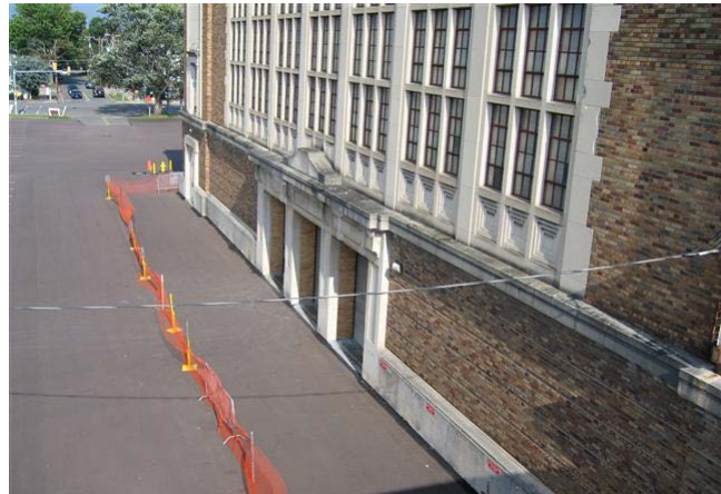
Fig. 2. Area cordoned off because of falling stone pieces.
