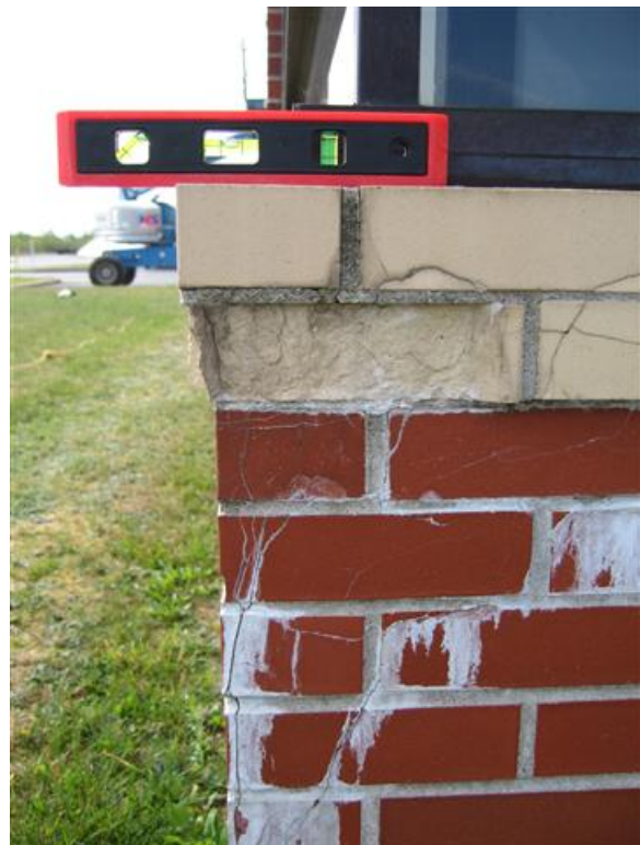
Fig. 9. Severely deteriorated masonry due to water infiltration at an improperly flashed window sill.
