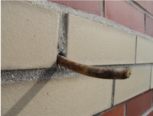
Fig. 8. Clogged weep tube keeps water trapped in the wall.
