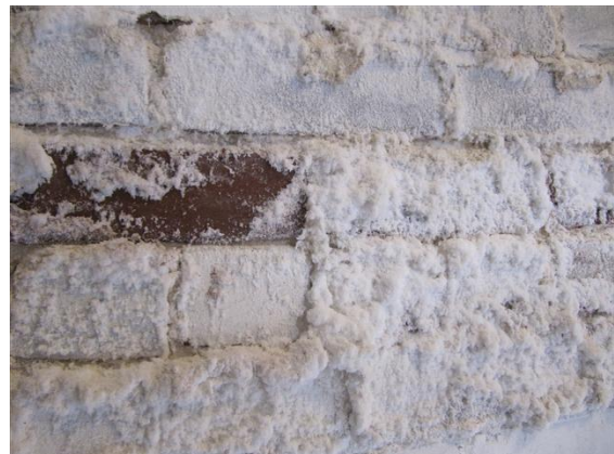
Fig. 1. Heavy efflorescence from re-crystallized salts.
