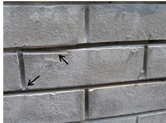
Fig. 7. Localized brick damage and partial mortar removal due to inadequate preparation.
