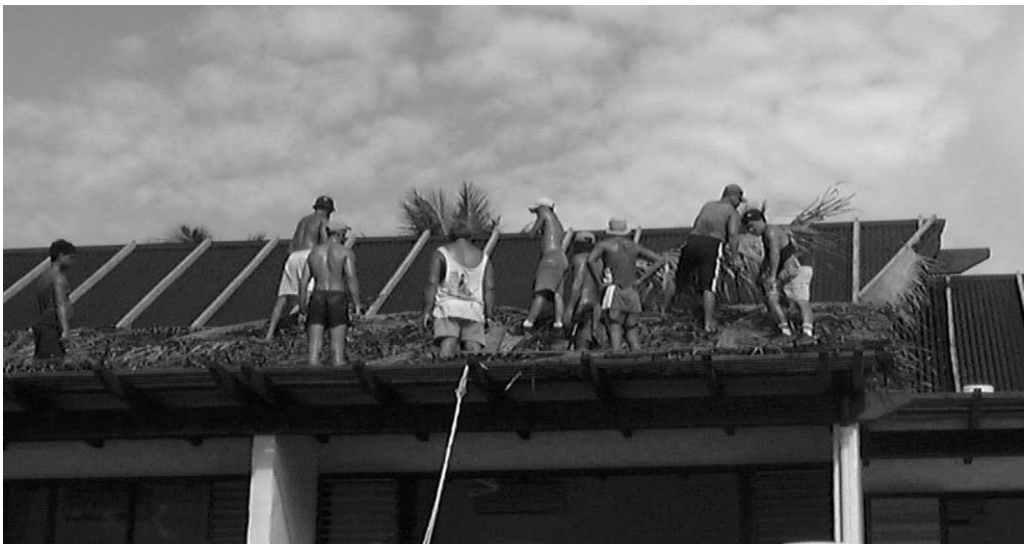
Figure 6.7 Thatched roofing project, South Pacific style. Can you find at least four violations of good safety practice?
