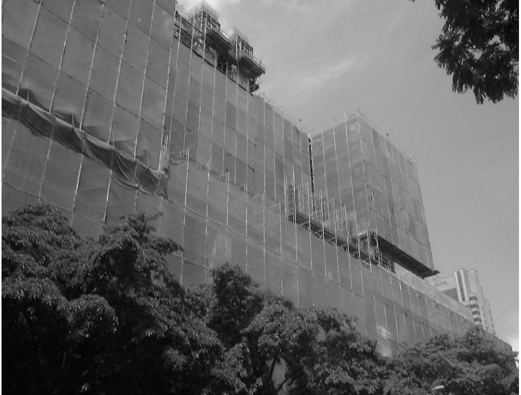
Figure 6.6 Safety netting on scaffolding, Singapore.
