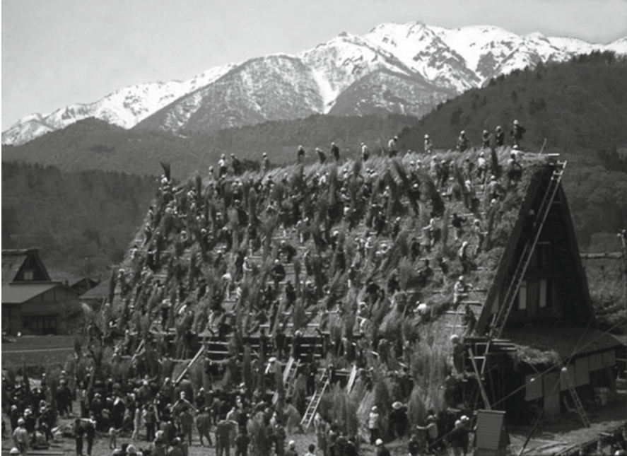
Fig. 10.1 Thatching the roof of a gassho-tsukuri , a traditional house in a Shirakawa village, Japan (Photo: provided by the Shirakawa village government)
