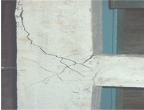
Fig. 8 Failure pattern of control specimen
