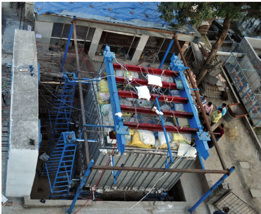
Fig. 4 Top view of the test arrangement with compartmentalization
