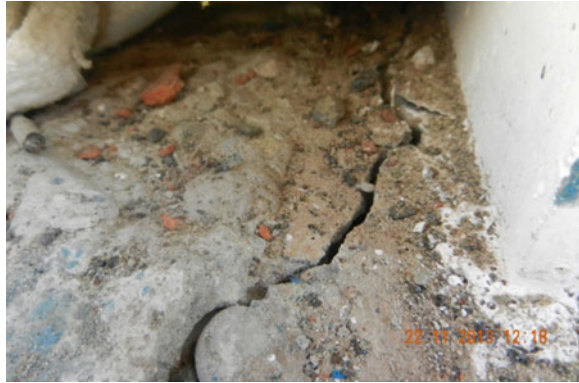
Fig. 9 A 6 mm wide crack measured on slab
