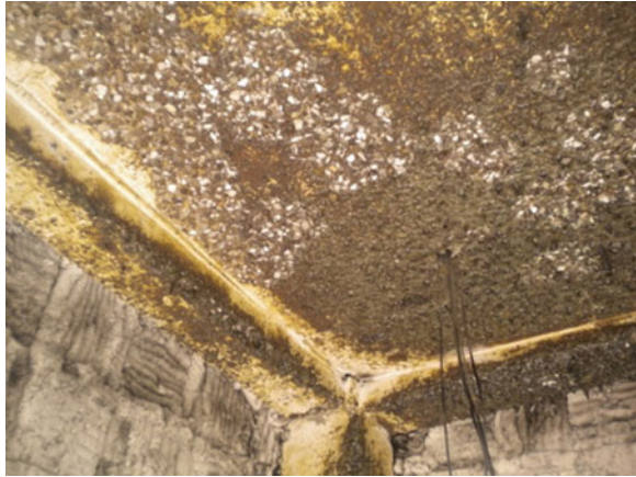
Fig. 12 Post fire view of the slab
