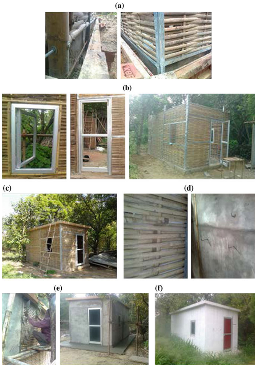
Fig. 6 Installation of wall panel and completion of bamcrete house at IITD. a Fixation of bamboo panel in concrete. b Installation of windows and door fittings. c Bamboo wall panels before mortar plaster. d Insertion of anchorages. e Mortar plastering of bamboo panels. f Bamboo concrete house
