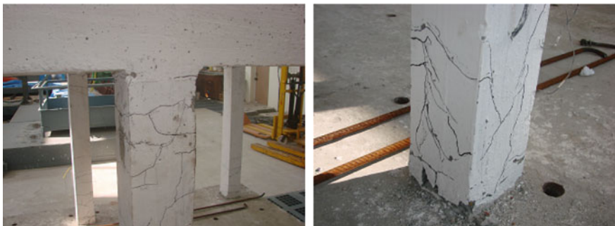
Fig. 9 Crack pattern in the ground storey columns
