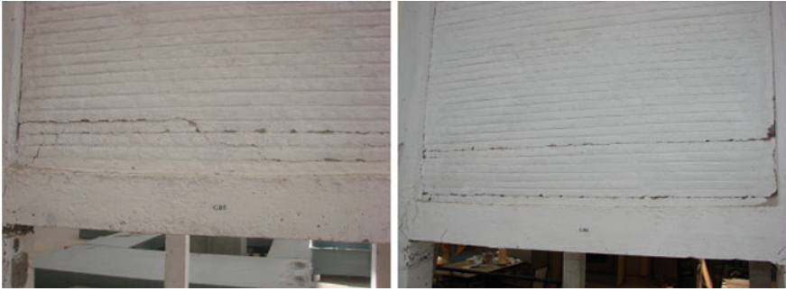
Fig. 10 Failure crack pattern of brick-infill wall panels of open ground storey building
