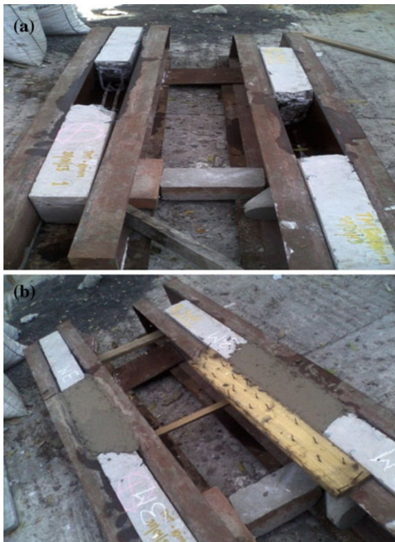
Fig. 2 a RPPC beam before retrofitting, after removing spelled concrete. b Beam after retrofitting
