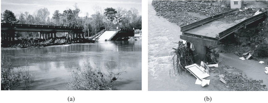
Fig. 1. Span blockage accumulation bridge failure. (a) Louisiana, USA, (b) Gangwon province, Korea.
