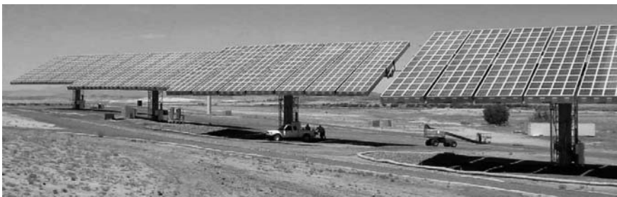
FIGURE 20.39 Several 35-kW Amonix modules installed in an Arizona Public Service power plant. The pickup truck underneath the module gives an idea of the scale.
