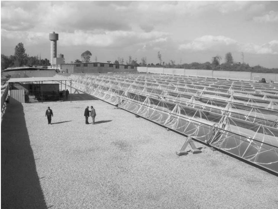
FIGURE 18.37 El NASR Pharmaceutical Chemicals, Egypt. Installed capacity: 1.33 MW th . (From Fichtner Solar GmbH, Germany. With permission.)
