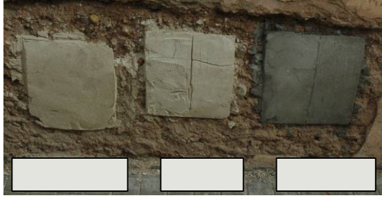
Figure 20: Mortar samples at the south façade.
