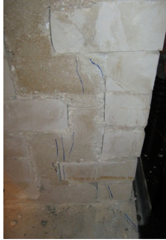
Crack initiation in W12
