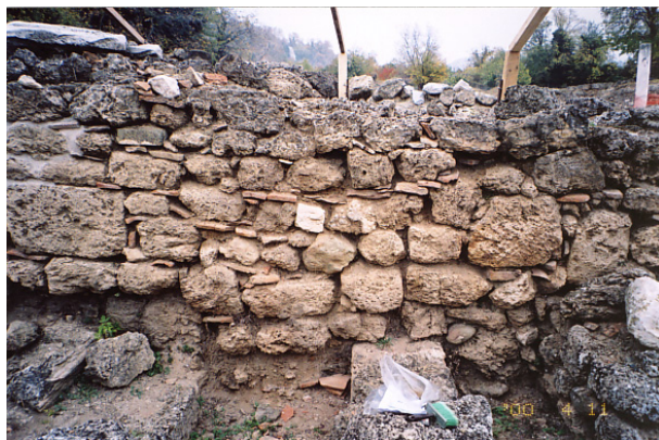
Figure 1: Absence of joints due to mortars' loosening.
