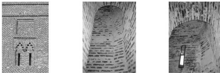
Figure 2: Aspects of the irregular mortar-brick disposition.
