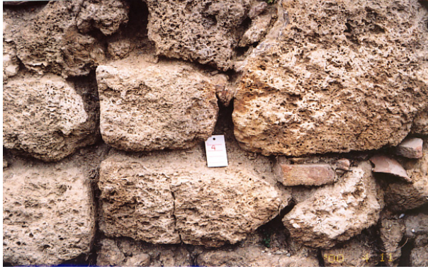
Figure 2: Cracks in stones.
