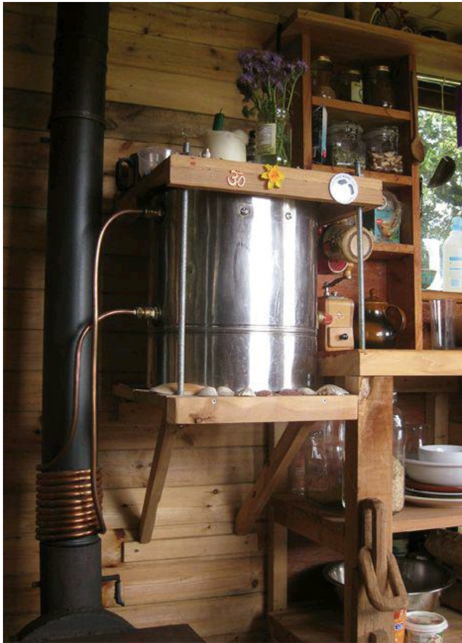
Noel's water heater uses the heat of the chimney to warm his water tank.
