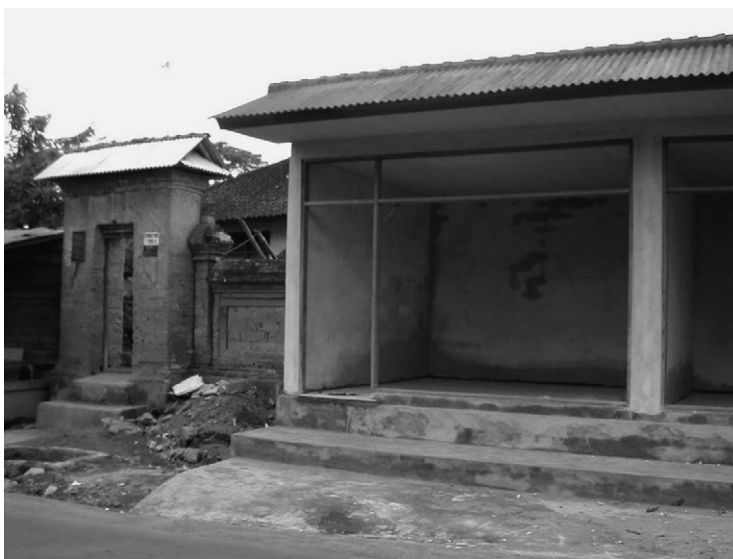
Fig. 5. Construction is Under Way for an Art Shop Located in Front of a Balinese Family Compound.
