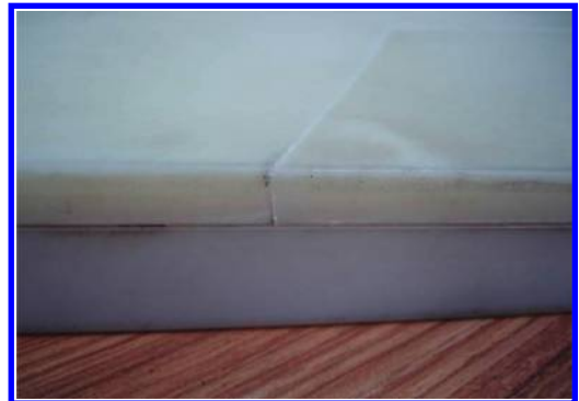
Figure 6. The experimental sample of cracks.
