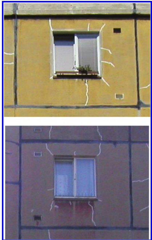
Figure 1. Distribution of real cracks in the external panel.
