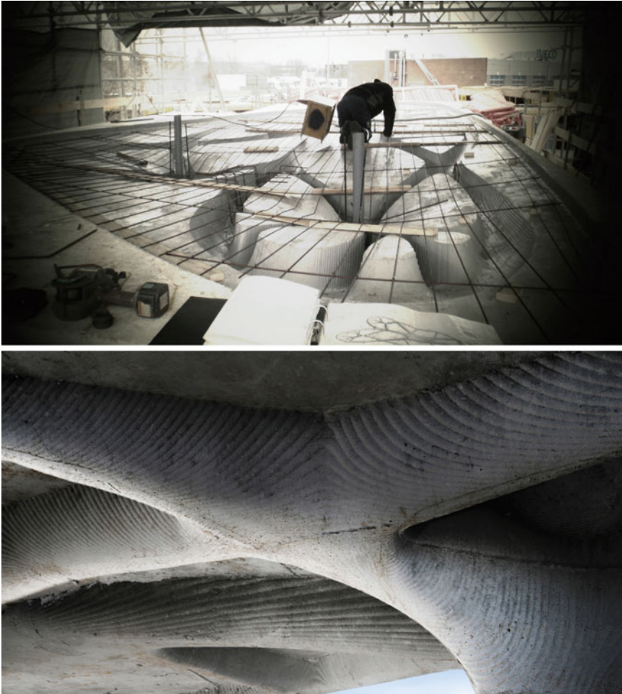
Fig. 3.20 CNC-milled casts were used for the manufacturing of the topologically optimized concrete structure of Unikabeton (Courtesy of Asbjørn Søndergaard)
