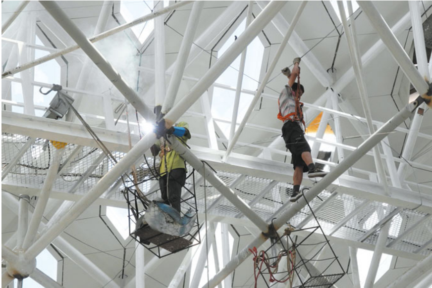
Fig. 4.30 The steel structure before installation of the inner skin (Courtesy of © Archivio Fuksas)
