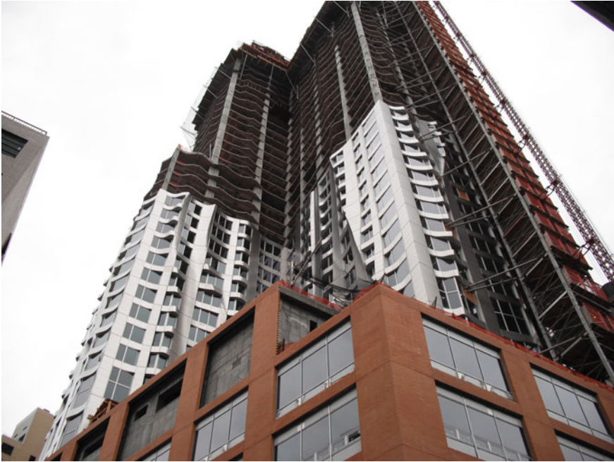
Fig. 4.16 Exact placement of 14,000 brackets of the curtain wall on the slab edges was required (Reproduced with permission of Permasteelisa Group)
