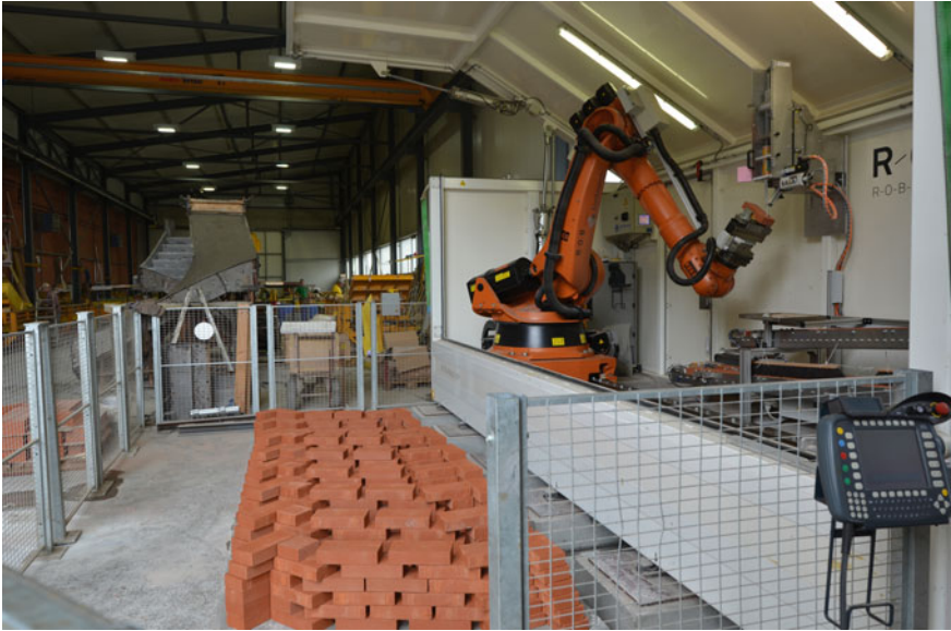
Fig. 4.7 Mockup construction: the robot is building the structures for supporting the diagonal elements (Reproduced with permission of © Gramazio & Kohler)
