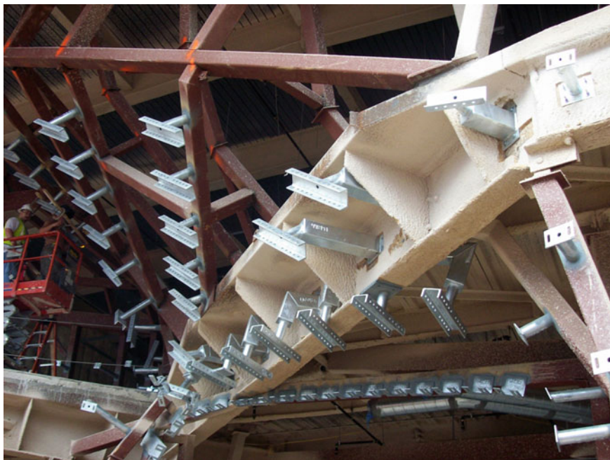
Fig. 4.42 Detail of the supporting steel structure showing the complexity that characterizes the interior space (© 2014 Method Design)
