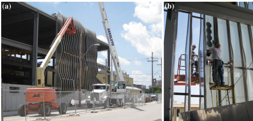
Fig. 4.14 a Façade aluminum components, installation (Reproduced with permission of Crawford Architects). b Façade glass components, installation (Reproduced with permission of Crawford Architects)
