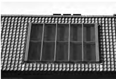
6.8 A roof-integrated solar air collector at Easthall, aligned with the glazed-in balcony
