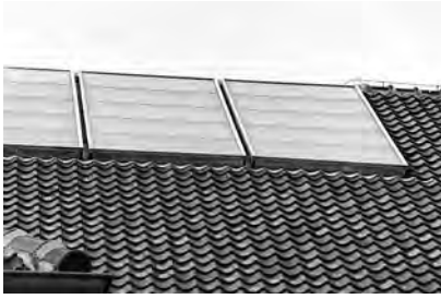
2.9 Detail of roof of swimming pool in Gouda – solar collector replacing former glazing
