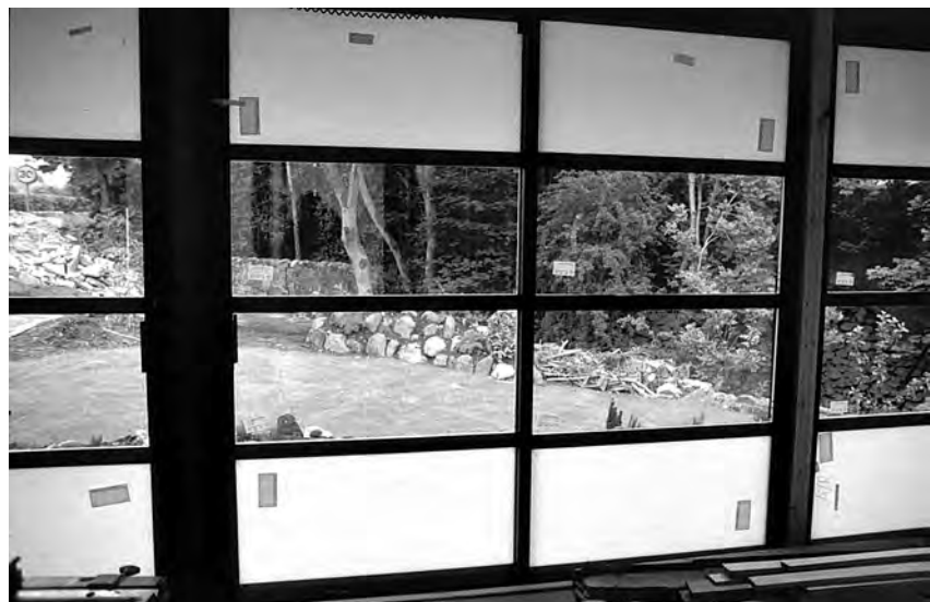
5.21 'Visi Heat' (clear) and 'Thermascrene' (translucent) glazing by Solaglas at Whalley house, under construction, June 1989 – note electric cable at extreme top of photograph
