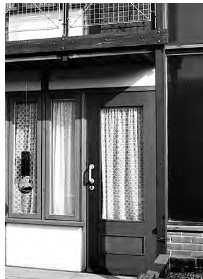
4.5 General view and close-up of south façade of Christopher Taylor Court – note prevalence of curtains for privacy on ground floor
