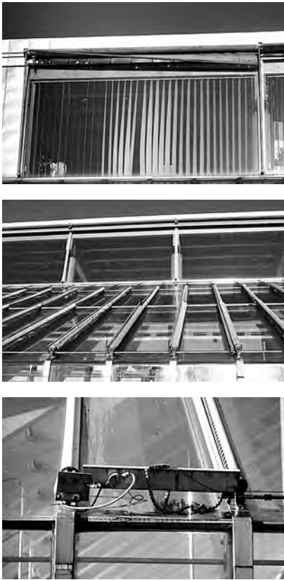
6.1 External shading mechanisms, Burrell Museum, Glasgow – these only operated for a short period relative to the life of the building (photographed November 2004)
